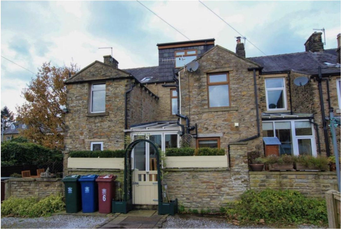
IMAGE SHOWING THE REAR OF N06 CLITHEROE ROAD DORMER AND OUTRIGGER ROOF ALTERATION
