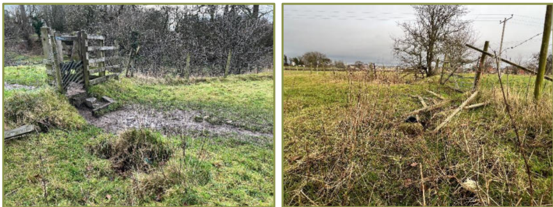
Left: Ø225mm culvert crossing under a public footpath. Right: Ø225mm Gated Field Access.
