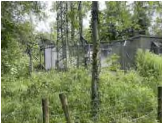
Photo 4— Mast and associated electrical infrastructure off site to the east
