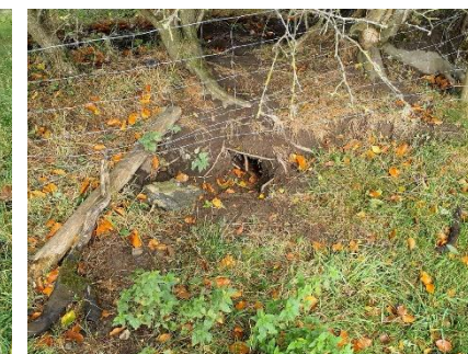
Figure 40 Hole under H08.
