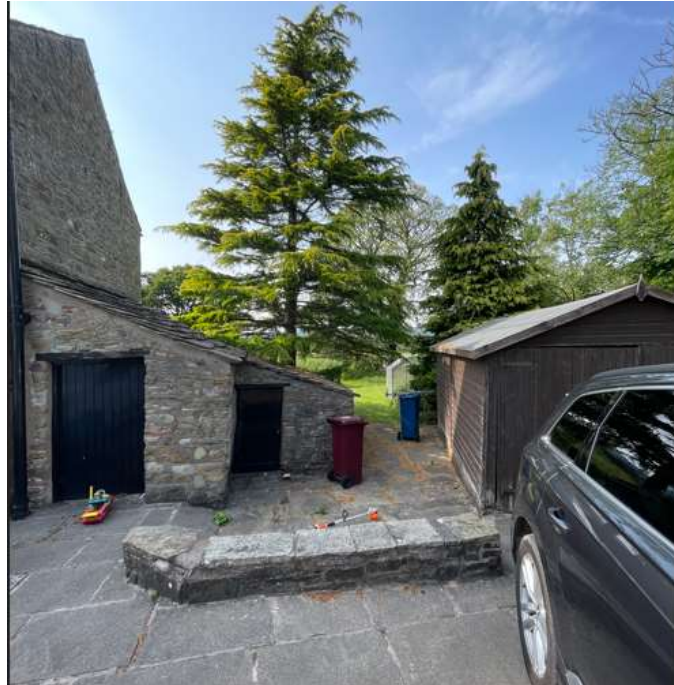
Dilapidated Workshop, Coal Store and External Timber Garage (to be replaced with new double Garage)
