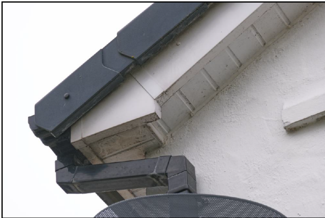
Image showing example of sealed soffit and roof edging with no potential access for birds or bats
