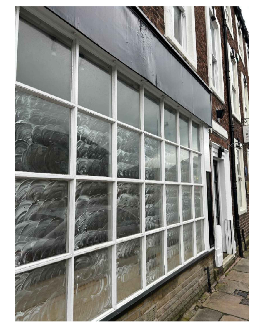
Existing External Photo - single glazed window with timber sill.
