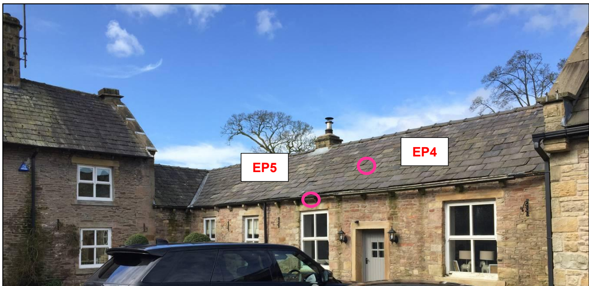
Figure 4.5 – Location of Emergence Points 4 & 5 on north-eastern roof pitch (EP4 & EP5)
