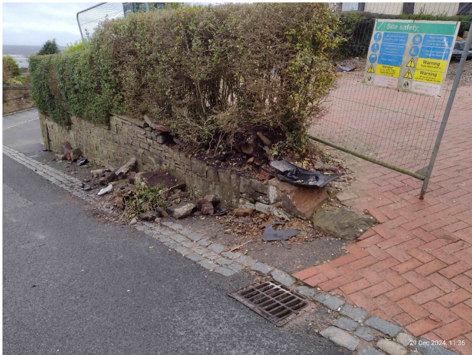
The wall after the vehicle damage December 2014
