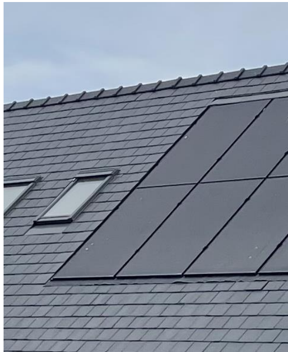
Pl. 1 Photograph showing an example of a new Spanish Blue slate roof with recessed Velux rooflights and black- framed recessed PV solar panels
