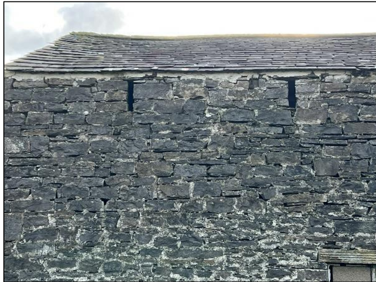
Photo 4: West elevation showing gaps to the pointing, and under the eaves and roof tiles.
