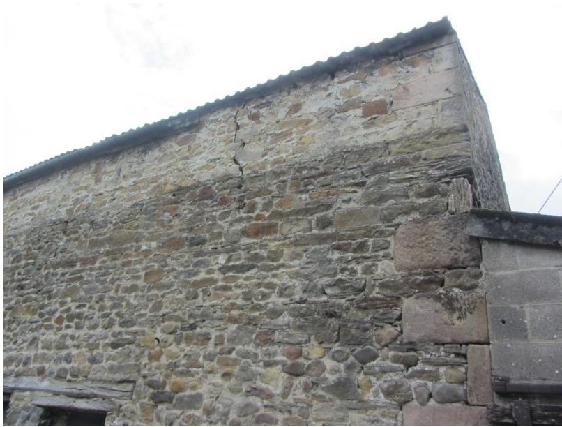
Photo 33 – Barn 2 – cracking in north wall
