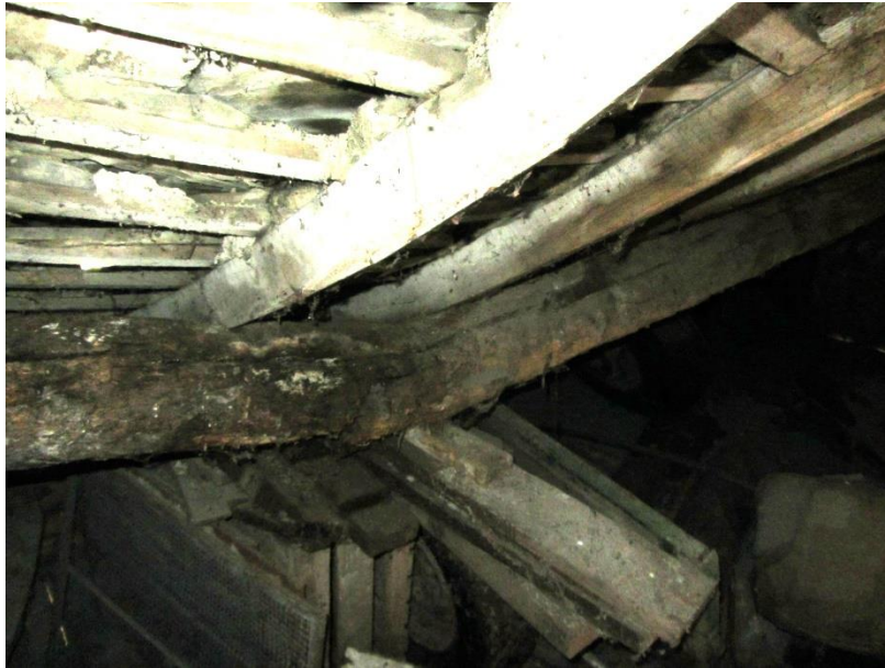
Photo 37 – Barn 3 – fractured purlin
