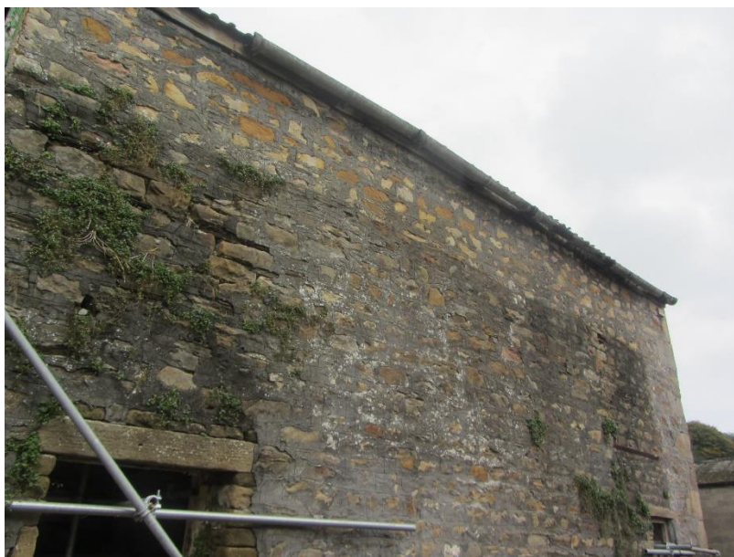
Photo 30 – Barn 2 – cracks and step in south wall
