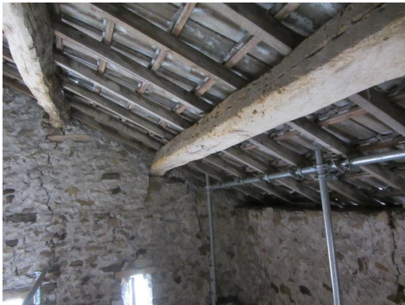
Photo 28 – Barn 2 – cracking in north and west walls
