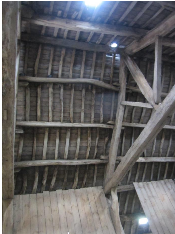
Photo 11 – Barn 1 – warped rafters and purlins
