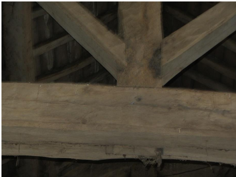
Photo 12 – Barn 1 – insect decay to roof truss
