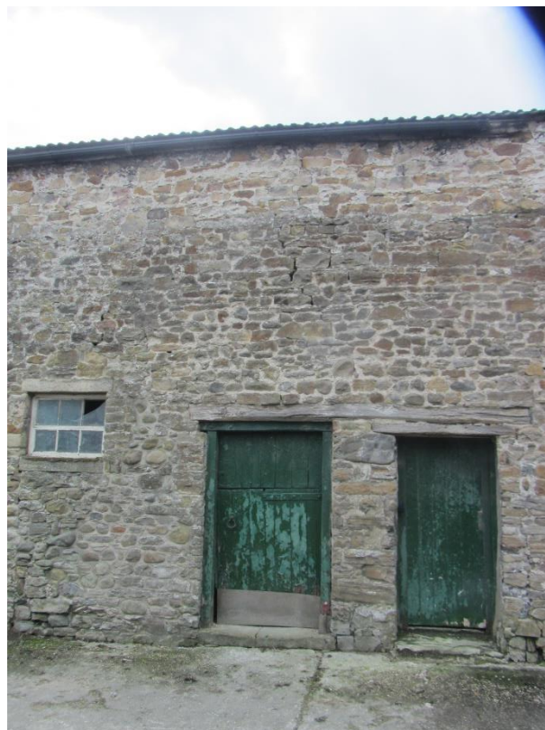
Photo 34 – Barn 2 – cracking in north wall
