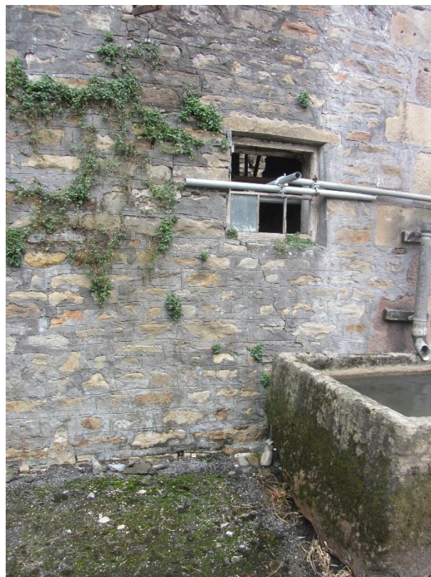
Photo 32 – Barn 2 – cracking in south wall
