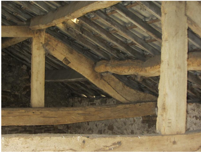
Photo 25 – Barn 2 – decayed roof timbers
