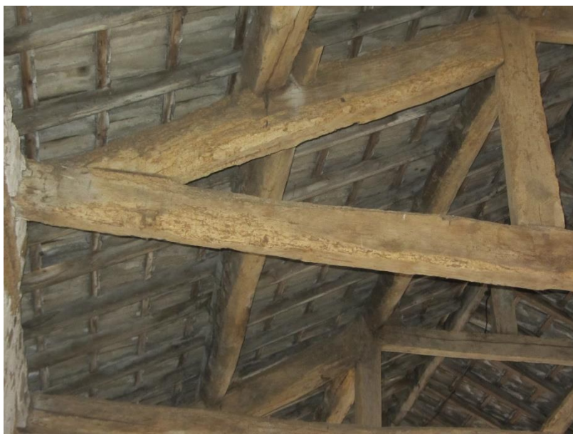
Photo 24 – Barn 2 – decayed roof timbers
