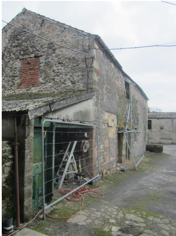
Photo 29 – Barn 2 – distorted and propped south wall
