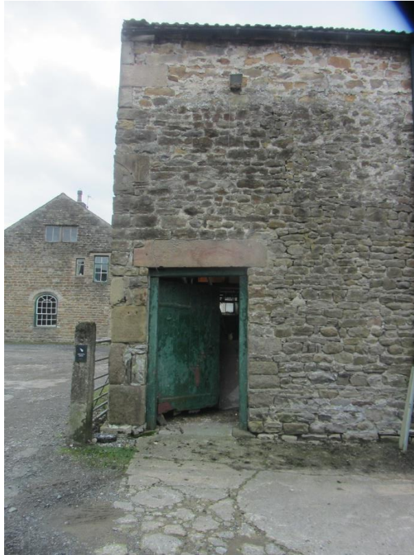
Photo 35 – Barn 2 – cracking in north wall
