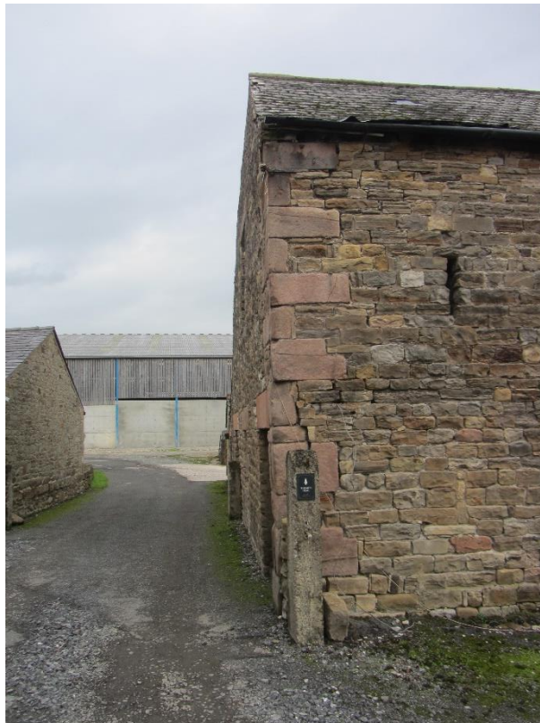
Photo 22 – Barn 1 – outward bulge in west wall
