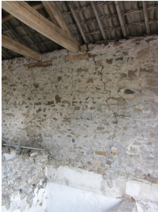
Photo 27 – Barn 2 – cracking in north wall
