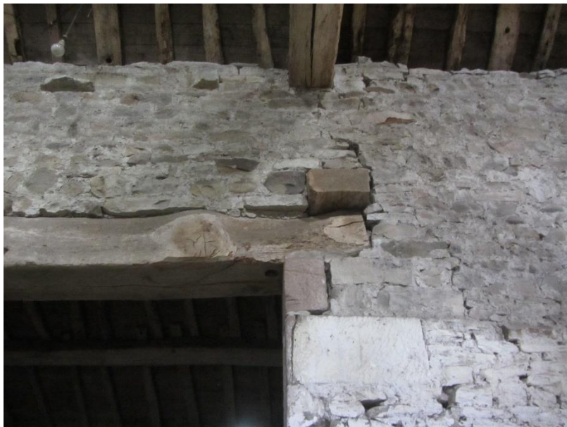
Photo 20 – Barn 1 – decayed lintel and cracks in wall
