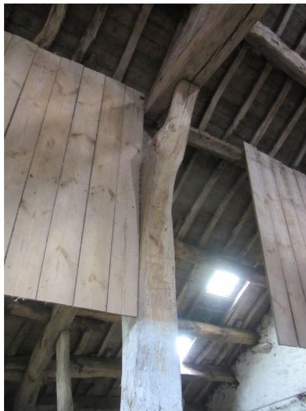
Photo 14 – Barn 1 – insect decay to timber post
