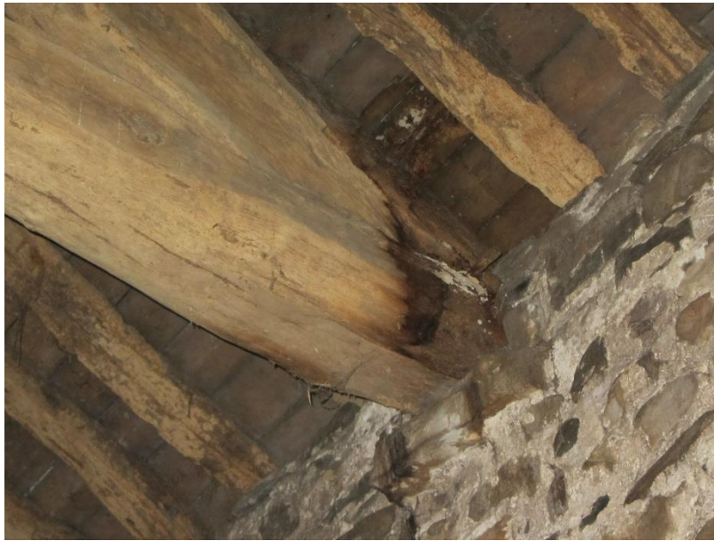
Photo 13 – Barn 1 – wet-rot at truss bearing
