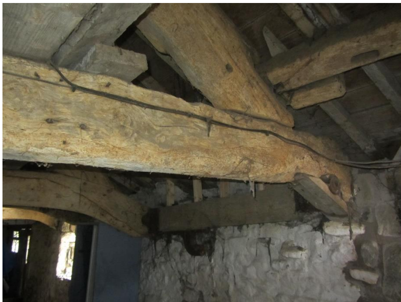
Photo 16 – Barn 1 – insect decay to shippon roof truss
