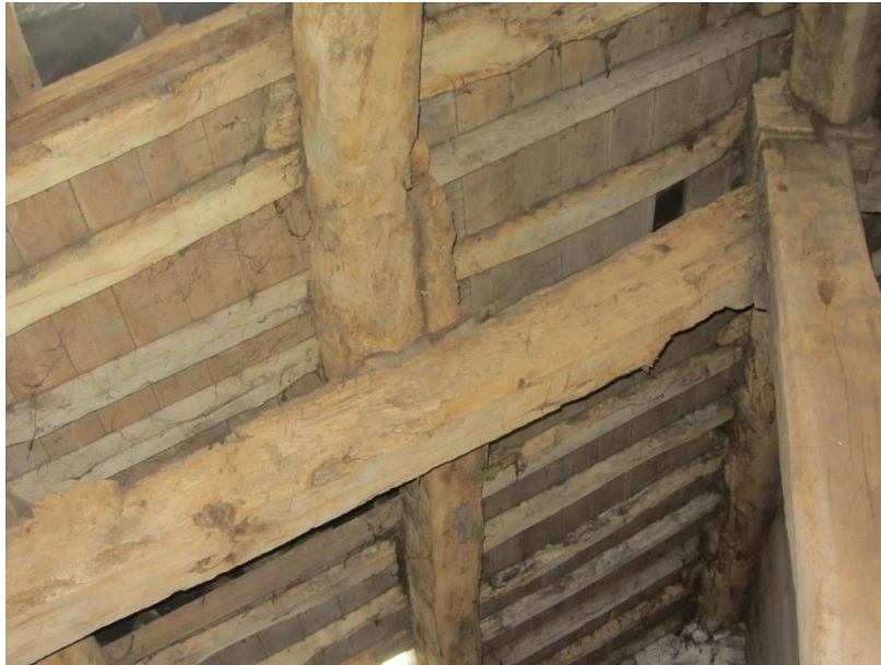
Photo 15 – Barn 1 – insect decay to shippon roof timbers
