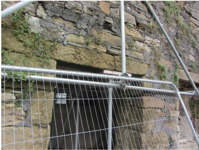
Photo 31 – Barn 2 – cracked lintel in south wall
