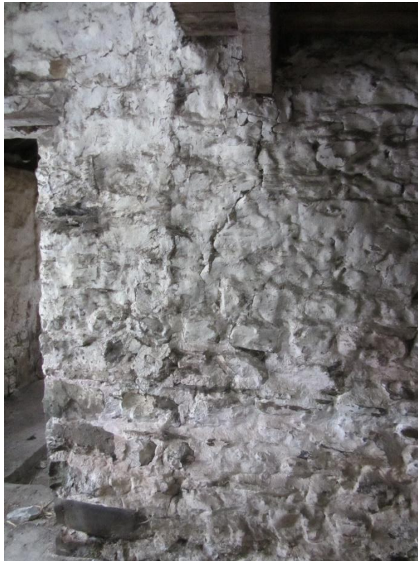
Photo 19 – Barn 1 – crack in internal wall
