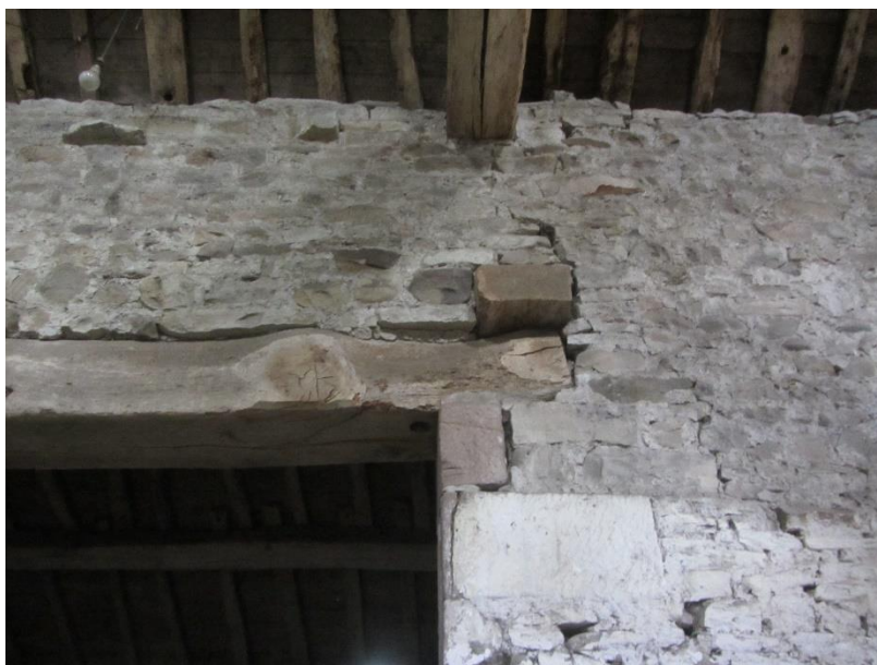
Photo 20 – Barn 1 – decayed lintel and cracks in wall
