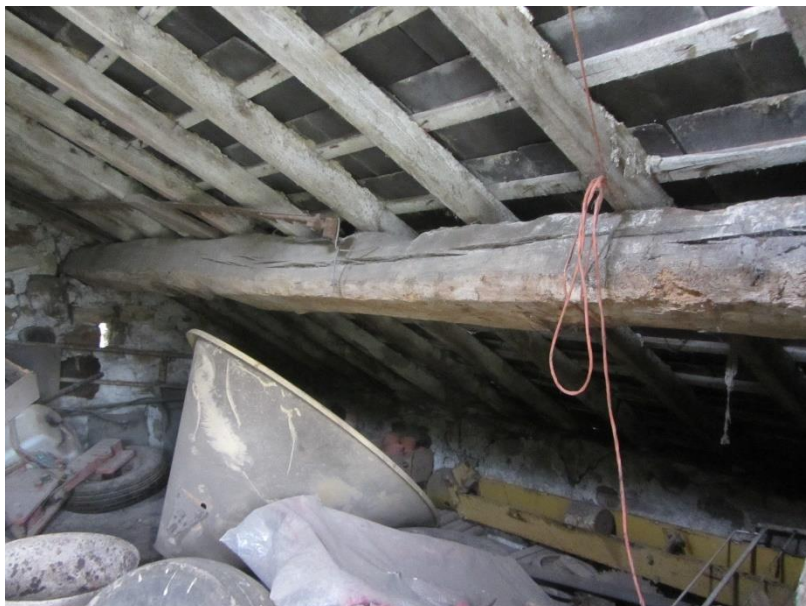
Photo 38 – Barn 3 – decayed roof timbers
