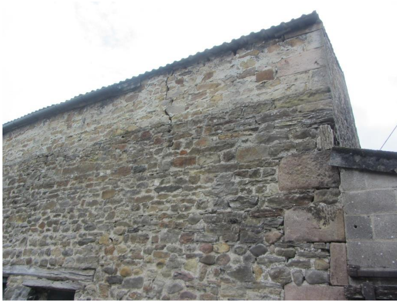
Photo 33 – Barn 2 – cracking in north wall
