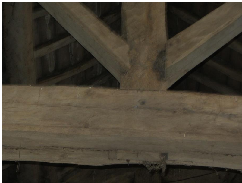
Photo 12 – Barn 1 – insect decay to roof truss
