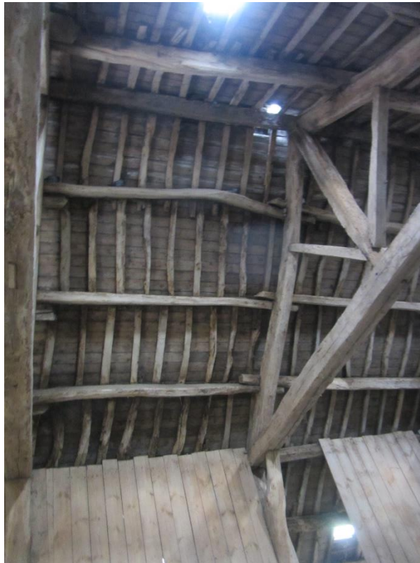
Photo 11 – Barn 1 – warped rafters and purlins
