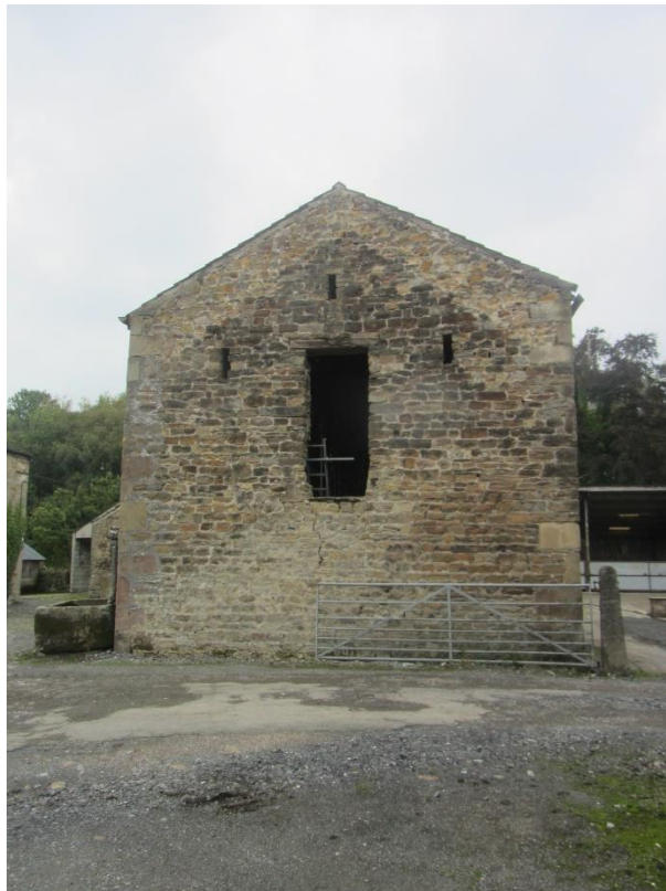
Photo 36 – Barn 2 – cracking in east wall
