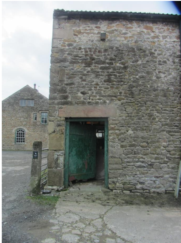
Photo 35 – Barn 2 – cracking in north wall
