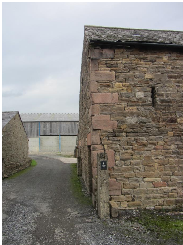
Photo 22 – Barn 1 – outward bulge in west wall
