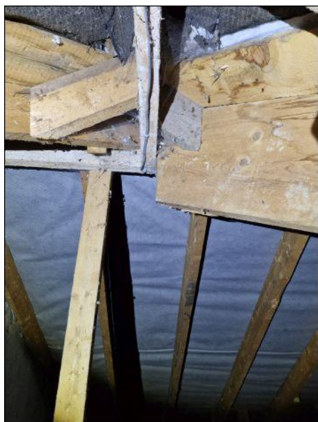
Photo 20: Roof beams above large aggregation of droppings in western roof void
