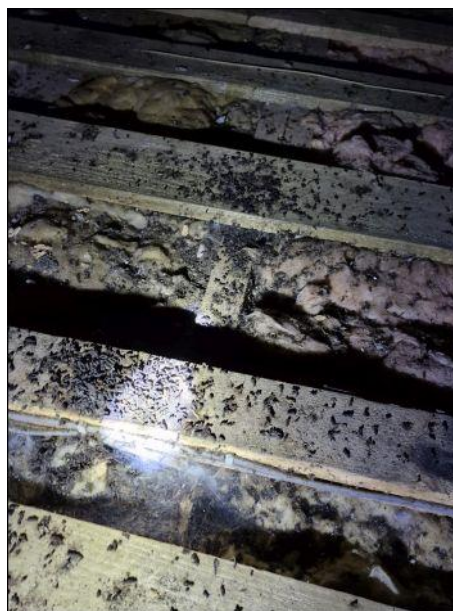
Photo 21: Mix of very old, old and more fresh droppings in western roof void
