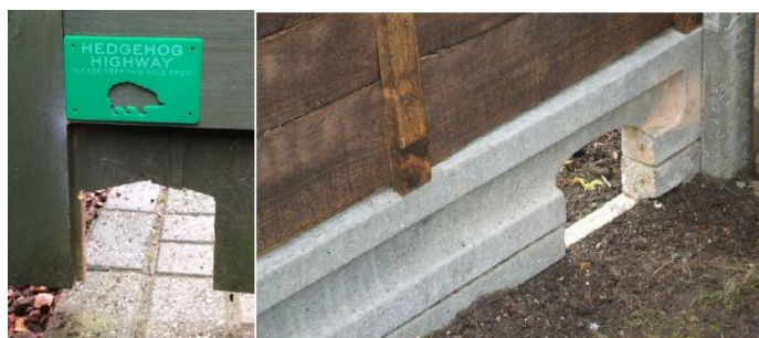
Insert 4: Showing wildlife access gap within fencing
