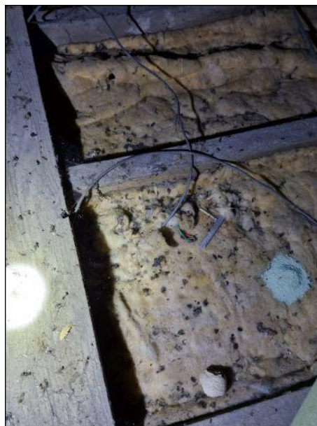
Photo 19: Scattered droppings in eastern roof void
