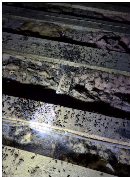
Photo 22: Mix of very old, old and more fresh droppings in western roof void
