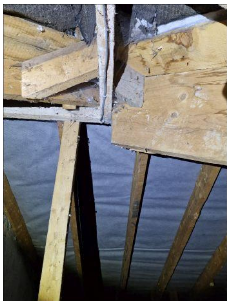
Photo 21: Roof beams above large aggregation of droppings in western roof void
