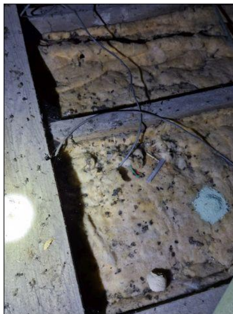
Photo 20: Scattered droppings in eastern roof void
