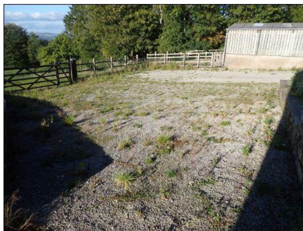
Photo 10: Vegetation colonising hardstanding
