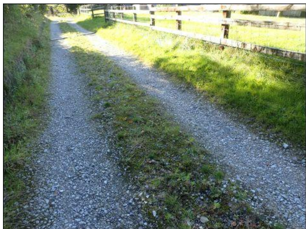
Photo 11: Vegetation colonising hardstanding
