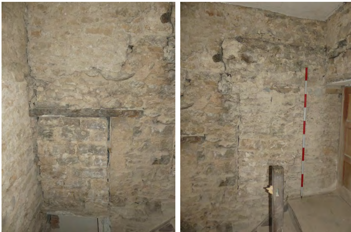
Plate 57 (left): Blocked landing-level doorway, north-east side of the south-east elevation, Room F2, viewed from the north-west
