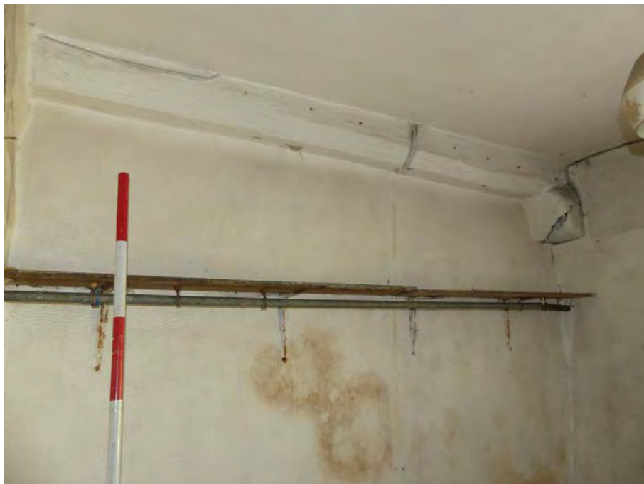
Plate 77: Beam at the north end of the west elevation of G5, viewed from the east
