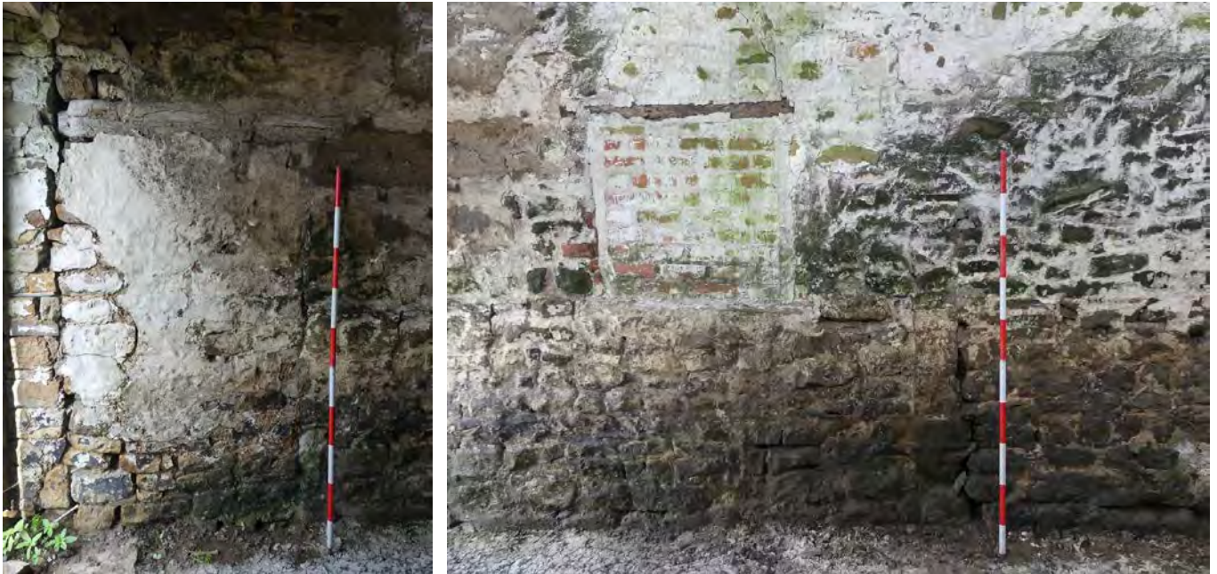
Plate 176 (left): Blocked door to the west side of the north elevation of G3, viewed from the south
