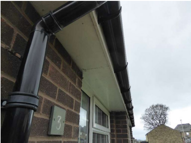
Front NW elevation showing soffit above ground floor window sealed tight to brickwork.
