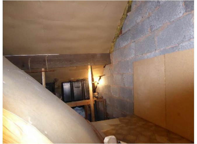
Storage space / loft to side of first floor bedroom, showing insulated roof lining boards.
