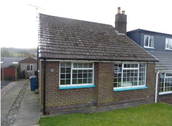
Front NW elevation, general view. All concrete roof tiles are tight fitting with no gaps or potential points of ingress for bats.
