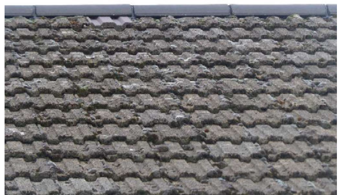
Rear SE elevation: all concrete roof tiles are tight fitting with no gaps or potential points of ingress for bats.
