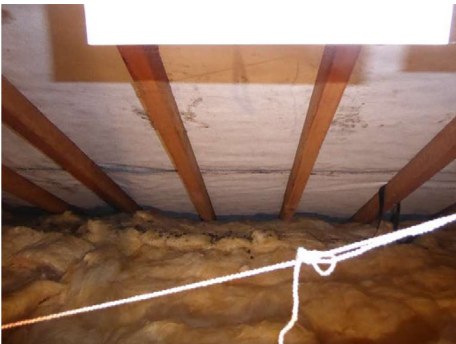
Storage space / loft to side of first floor bedroom, showing insulated roof lining boards.
