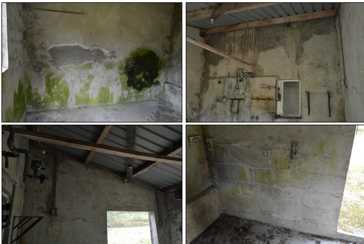
PL66: Views within the south unit of the west lean-to. Cracking and staining were widespread as well as algal growth and salt contamination / efflorescence which are suggestive of damp conditions. It is recommended that the plaster finishes are removed throughout the building. This will also allow for an assessment of the underlying wall fabric.
