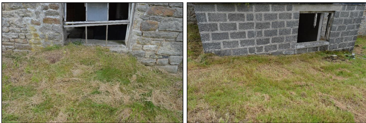
PL61: View of raised ground levels to the west elevation of the building.
