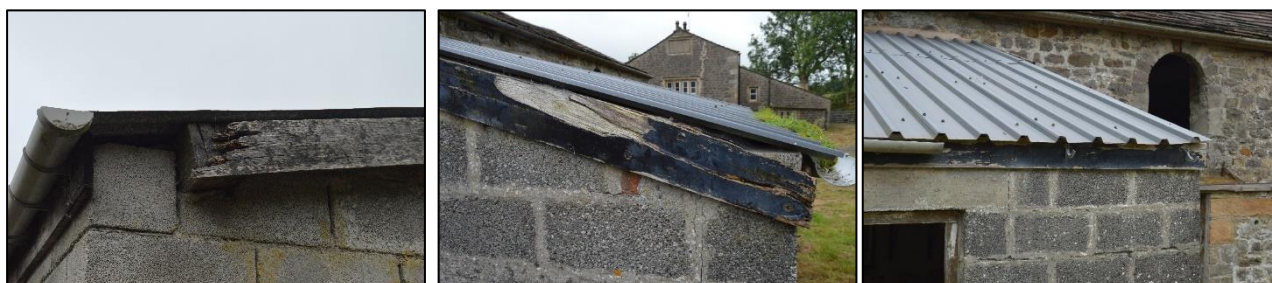
PL89: Evidence of decay noted to timber fascia boards.
