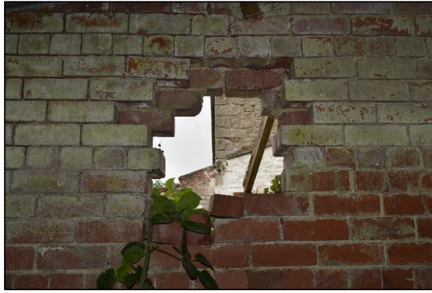
PL33: A hole was noted in the brickwork to the south wall of the north lean-to structure.
