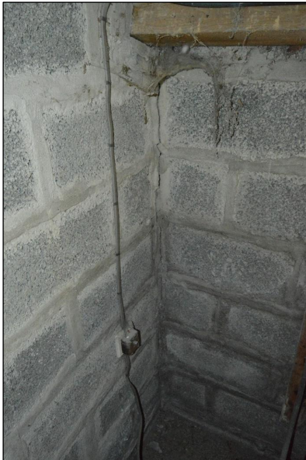
PL65: Isolated cracking noted to the west end of the internal wall within the north unit of the west lean-to. The cracking was deemed to be slight (between 1mm and 5mm) to moderate (between 5mm and 15mm) and likely occurred as a result of some
