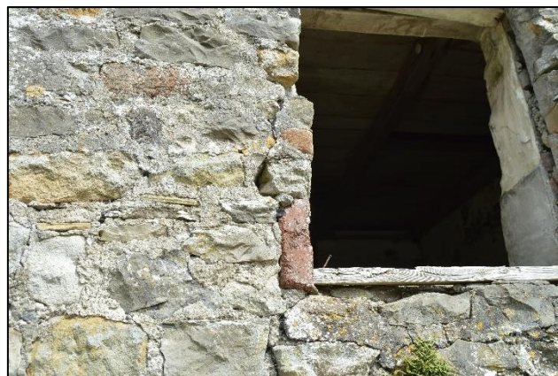
PL49: Loose / poorly consolidated masonry noted to the LHS jamb of the east window to the east window opening to the south gable end of the south addition. Making good is recommended.
