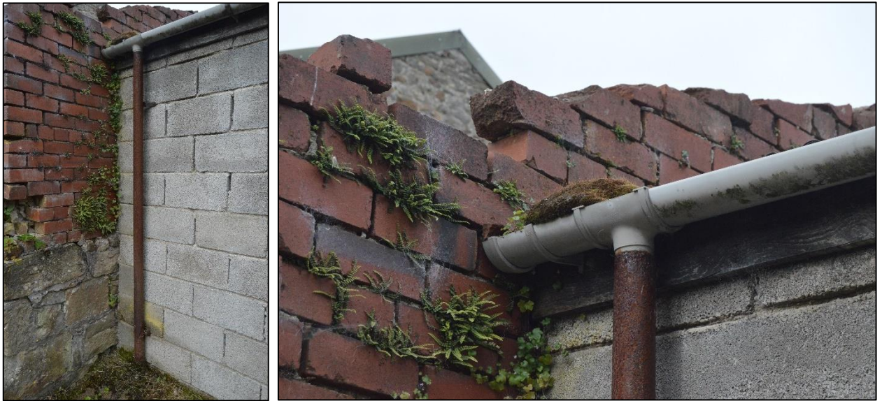
PL26: View of the existing rusted downspout to the east side of the north lean-to structure. Moss / plant growth was noted to the gutter outlet.
