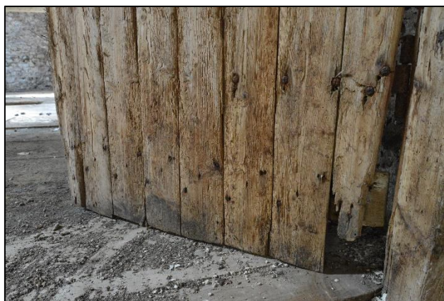
PL93: Evidence of decay and insect attack noted to the internal door to the south hay loft.
