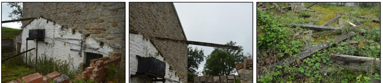
PL07: View of the now dilapidated and collapsed roof structure to the brick-built north addition.
