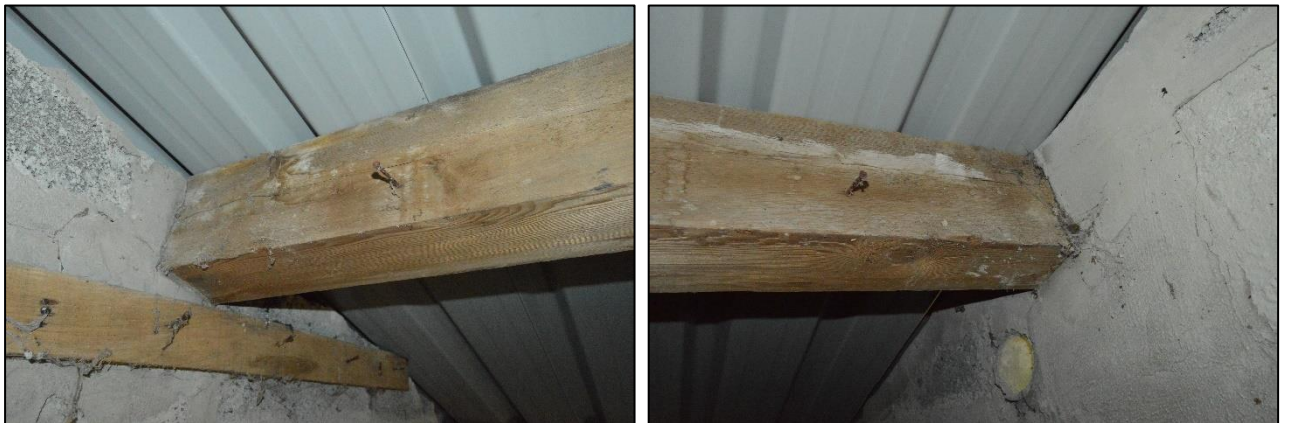
PL11: View of minor staining noted to the timber roof structure to the north side of the west lean-to structure.
