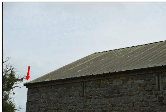
PL28: Plant growth noted to the west gutter to the main core of the barn.
