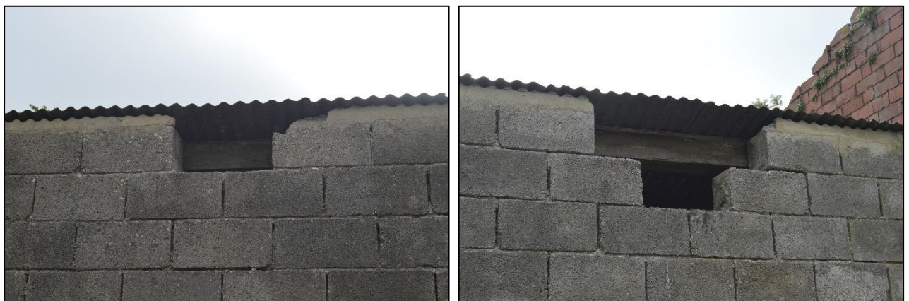
PL32: Missing blockwork noted to the west side of th north lean-to structure. It could not be confirmed if this is intentional but the exact purpose was not known at the time of inspection.
