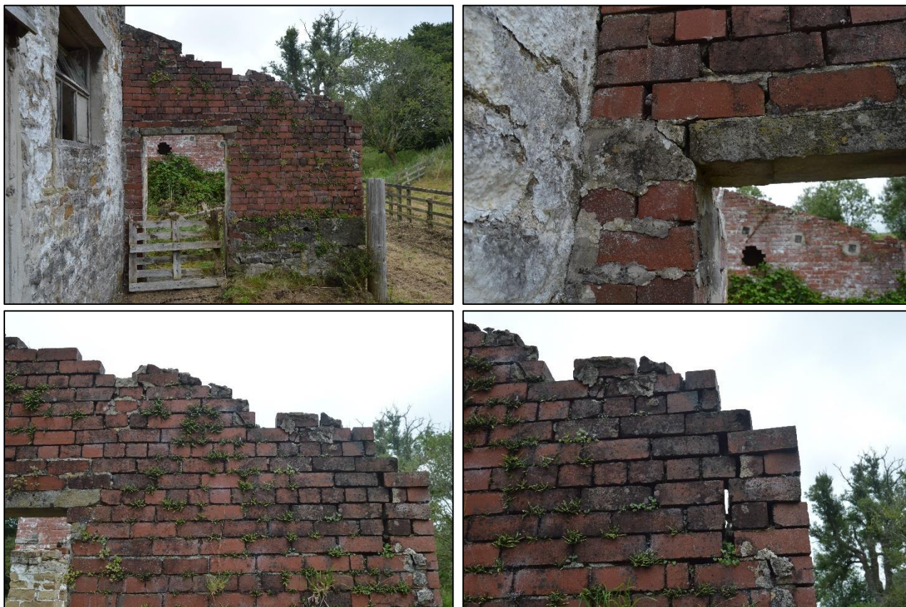
PL37: The masonry to the south east corner of the brick built north addition was loose and unconsolidated. The lintel to the door opening had virtually no end bearing onto the masonry below. The masonry is considered to be unsafe and is at risk of imminent collapse.
