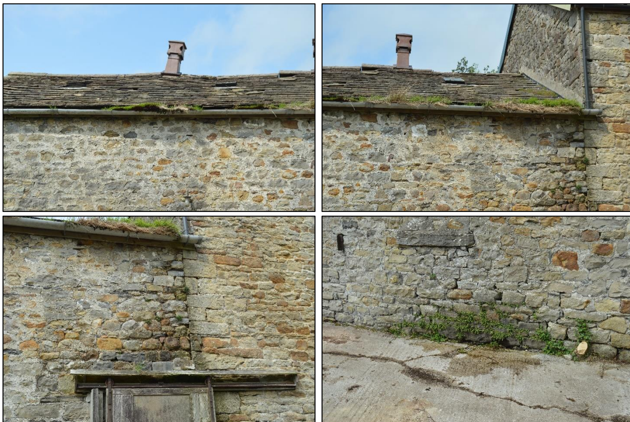
PL29: View of the significant plant growth to the guttering on the east side of the south addition. Wall staining and plant growth suggests the presence of leaks to the guttering as well as overflowing during periods of rainfall.
