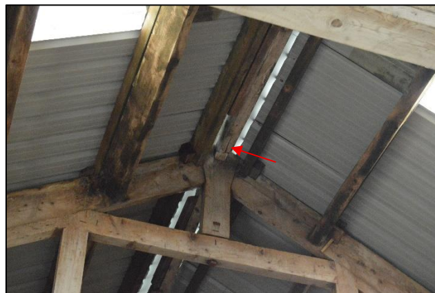
PLI 8: A shake / split was noted to the ridge at a location of a joint to the ridge beam of the roof to the main core of the barn. A closer assessment of this area is recommended on erection of a safe working platform to confirm the structural integrity of the ridge beam at this location. This being said, no obvious specific issues were identified at the time of inspection to suggest any immediate cause for concern, however a closer assessment is recommended to confirm.
