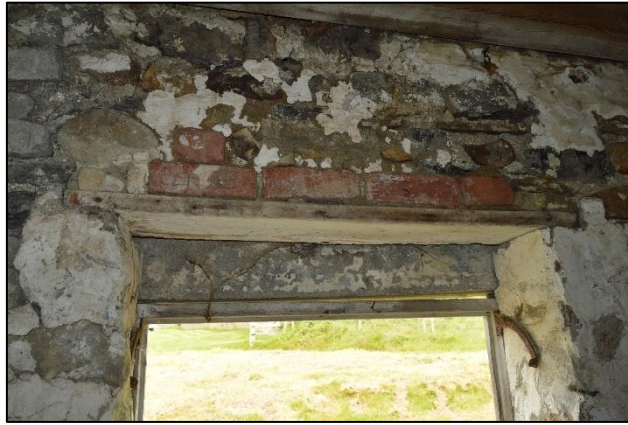
PL53: The lintel over the west opening present to the south end of the west elevation was noted as being slender with a minimal end bearing. It is recommended that the lintels are replaced with new lintels with a minimum end bearing of 150mm – 200mm.
