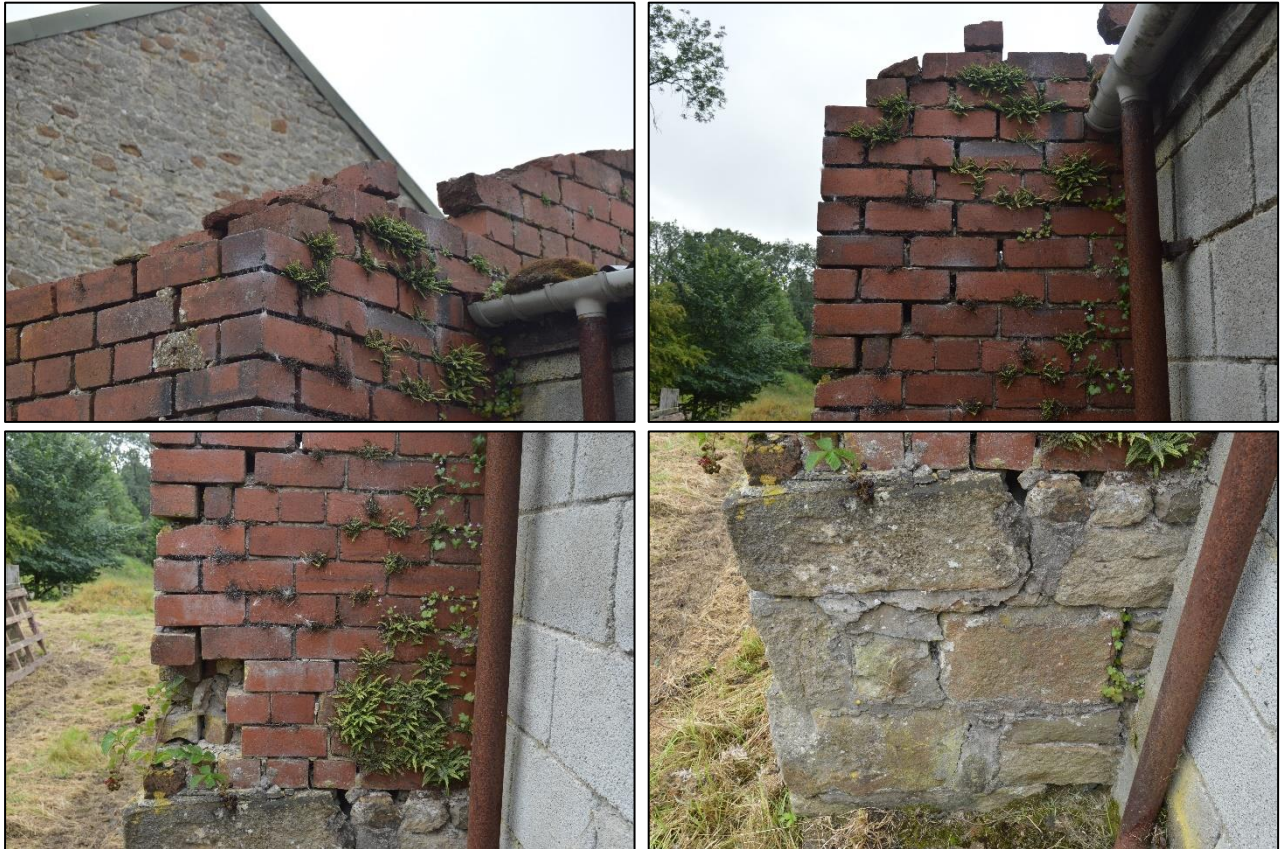
PL35: Loose and unconsolidated masonry noted to the north east corner of the brick built north addition.
