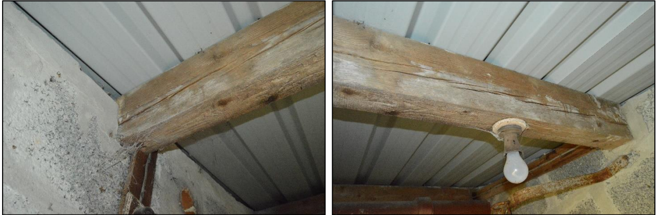
PL10: View of minor shakes noted to the timber roof structure to the north side of the west lean-to structure.
