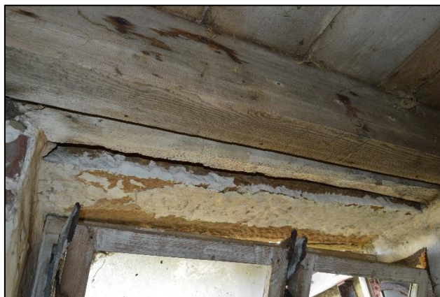
PL56: Evidence of wood-boring insect attack was noted, i.e. insect flight holes, to the timber lintel over the east elevation ground floor window of the south addition, adjacent to the west lean-to structure. It is recommended that the lintel is replaced.
