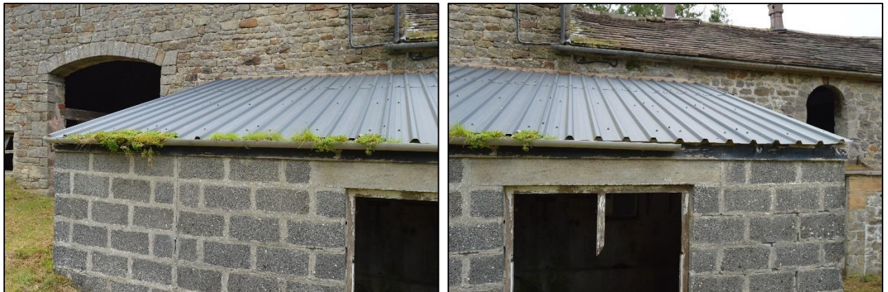
PL27: View of the plant growth to the gutter to the west lean-to structure as well as a missing section of guttering.
