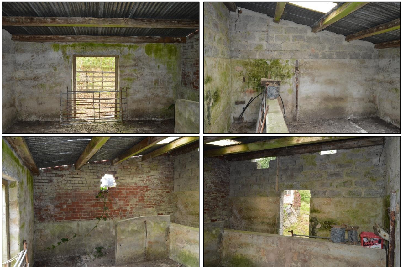
PL63: Internal views within the north lean-to structure. Cracking and staining were widespread as well as algal growth and salt contamination / efflorescence which are suggestive of damp conditions. It is recommended that the plaster finishes are removed throughout the building. This will also allow for an assessment of the underlying wall fabric.
