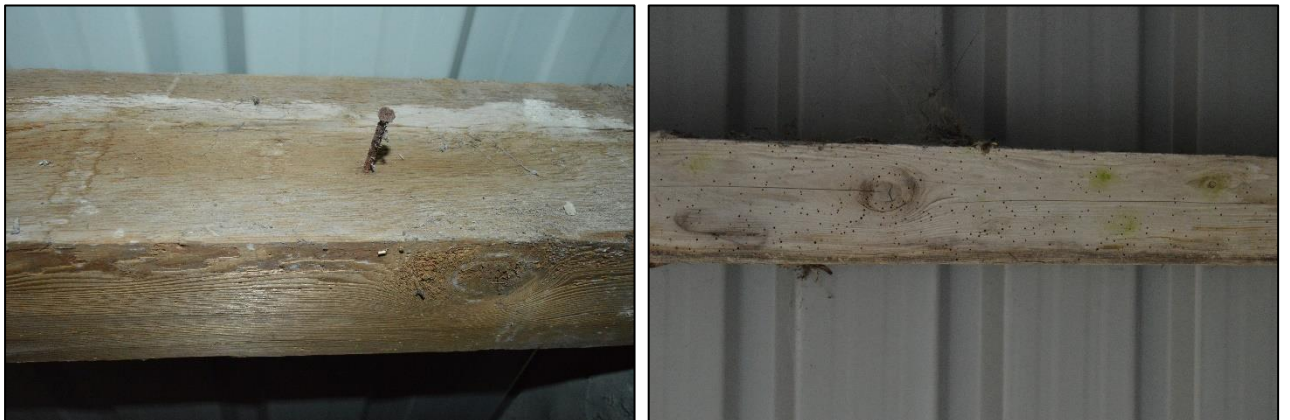
PL12: View of evidence of wood-boring insect attack i.e. insect flight holes, noted to the timber roof structure of the west lean-to structure.
