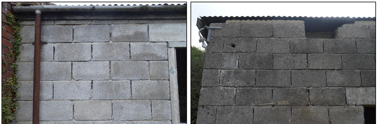
PL31: View of the degraded / missing pointing noted throughout the external walls of the north lean-to structure.
