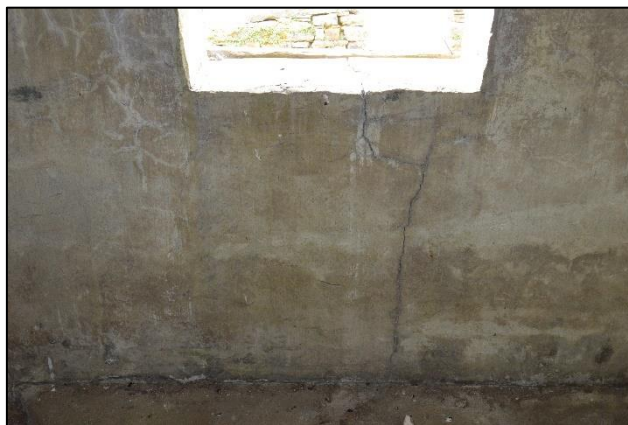
PL68: An isolated crack was noted to and below the cill to the east window of the south gable to the south addition. The cracking was deemed to be slight (between 1mm and 5mm). Cracking was also noted externally to the gable end above this particular window opening, however it could not be confirmed if this internal cracking was related at the time of inspection or if it is just superficial. Further investigations are recommended to confirm.
