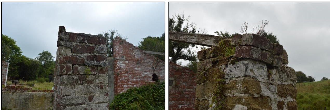
PL38: Loose masonry not to the top of the freestanding masonry columns within the brick built north addition
