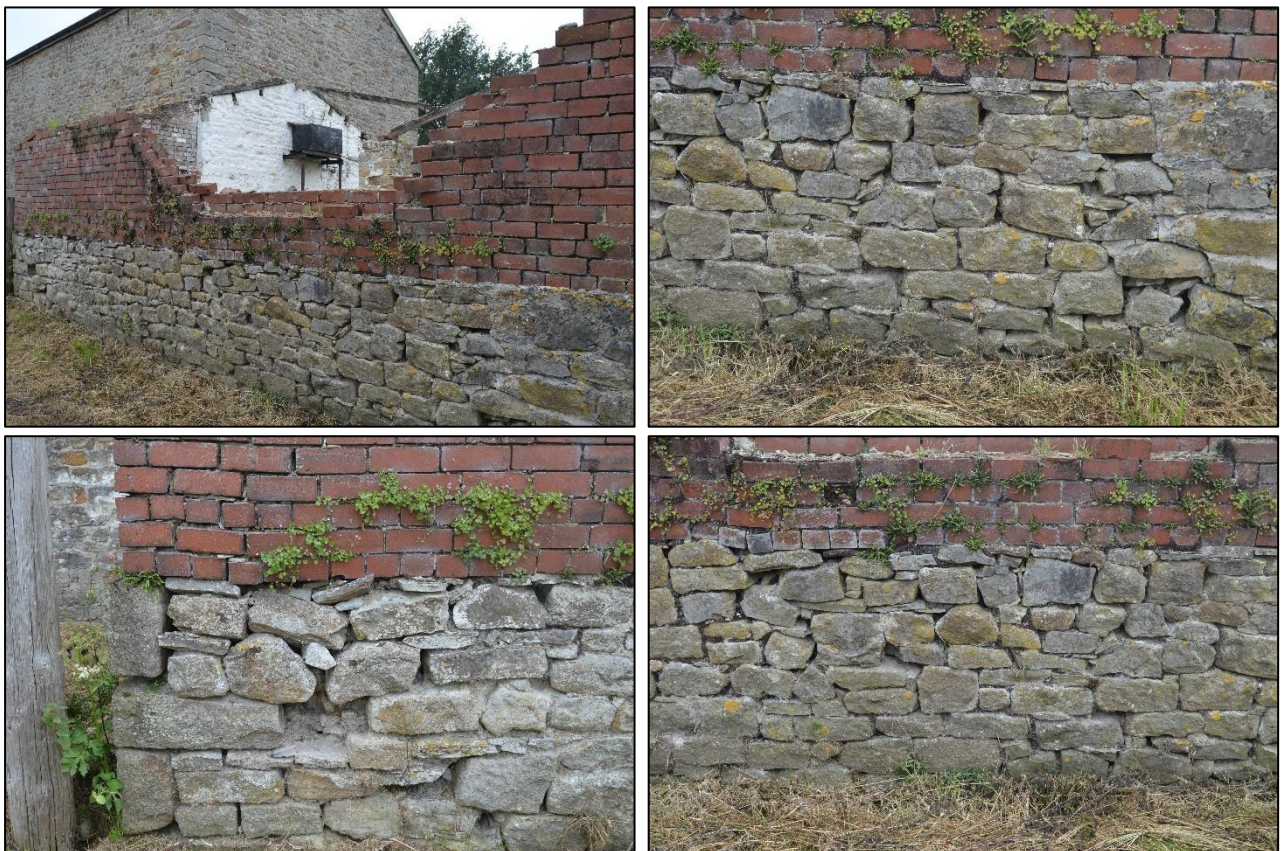
PL36: The remains of the east wall of the brick built north addition was leaning towards the east at the time of inspection. The masonry was largely loose and unconsolidated and is considered to be unsafe. The mortar to the pointing was largely perished.
