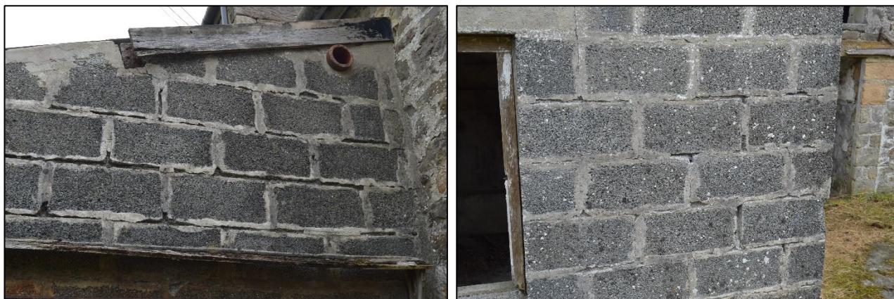
PL39: View of the degraded / missing pointing noted throughout the external walls of the west lean-to structure.
