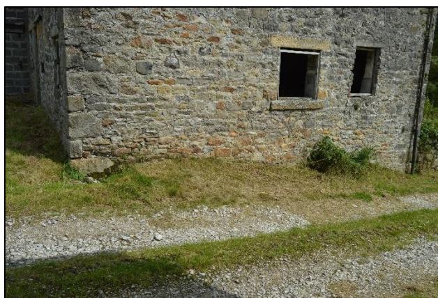
PL62: View of raised external ground levels to the south end of the building.
