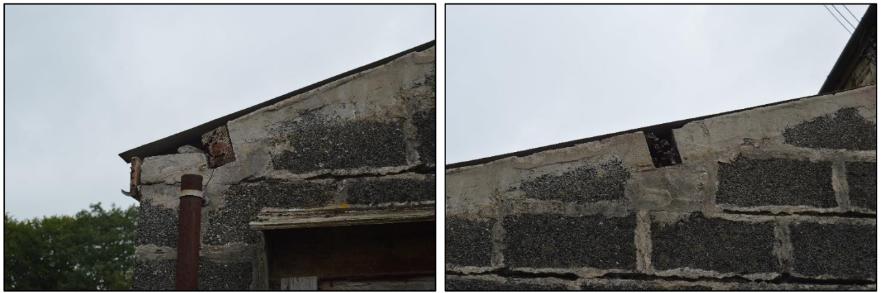
PL13: View of exposed and decayed purlin ends to the west lean-to structure.
