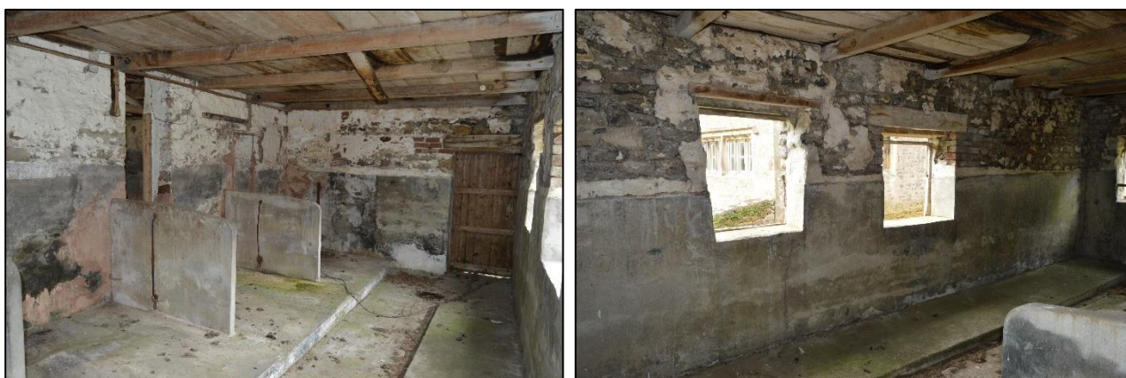
PL67: Views within the south shippon to the south addition. Cracking and staining were widespread as well as algal growth and salt contamination / efflorescence which are suggestive of damp conditions. It is recommended that the plaster finishes are removed throughout the building. This will also allow for an assessment of the underlying wall fabric.
