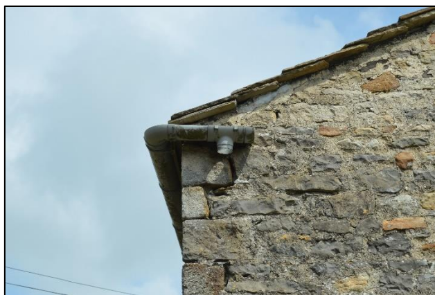
PL30: View of missing down spout to the south west corner of the south addition.
