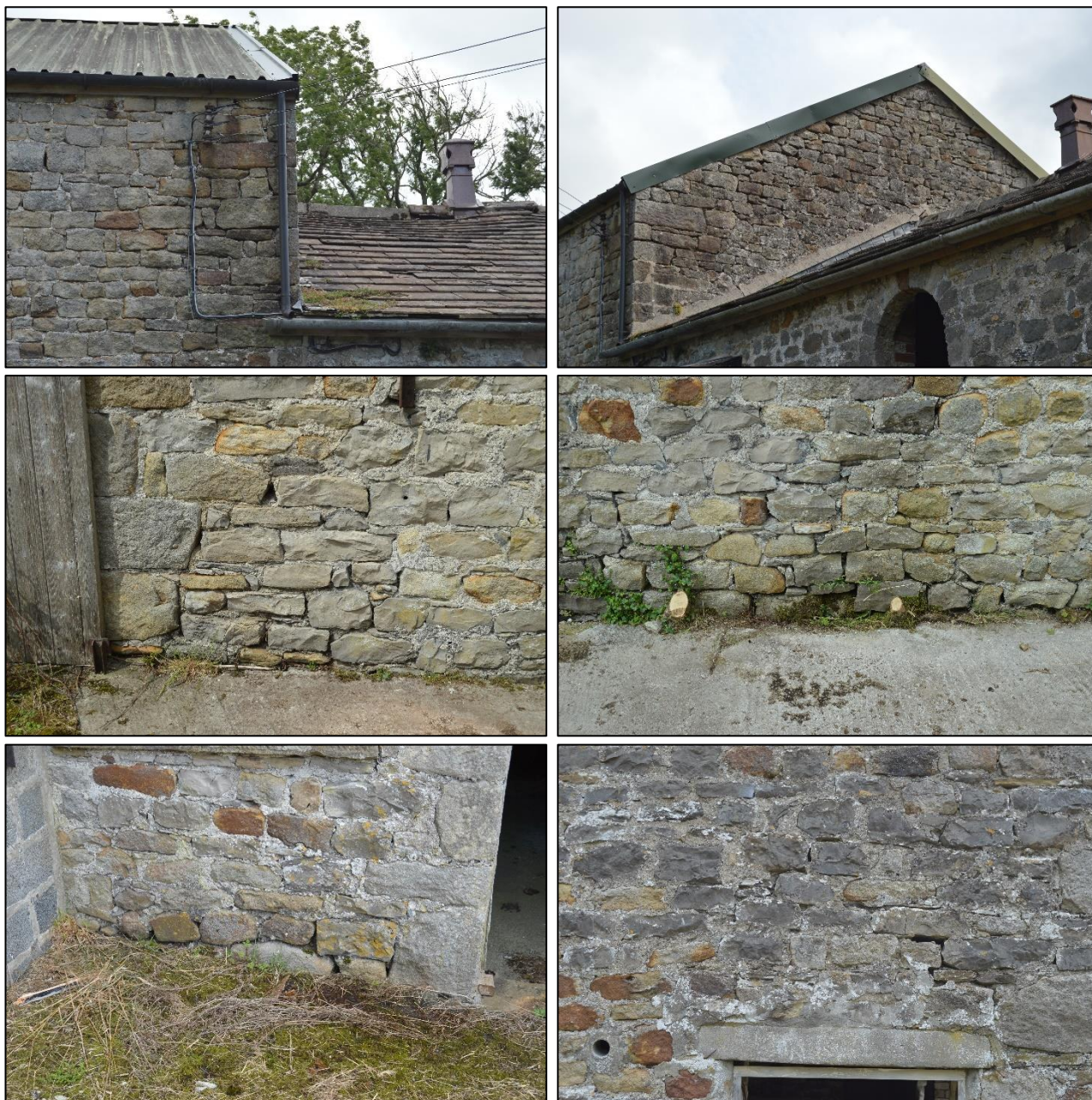
PL42: Areas of perished mortar was widespread throughout the building and repointing is recommended using a lime mortar.
