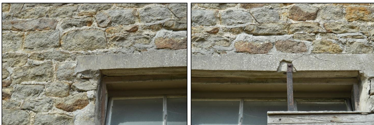
PL43: Cracking noted to the lintel to a window to the ground floor of the east elevation of the main core of the barn. The front of the lintel appeared to be comprised of a cement veneer and it could not be confirmed if it was only the veneer was cracked or if the crack was also present the underlying structural support, the type, condition and adequacy of which could not be confirmed at the time of inspection.
