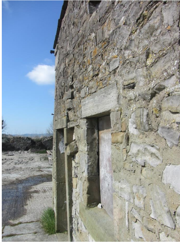
Photo 19 – South corner – cracked and bulging stone
