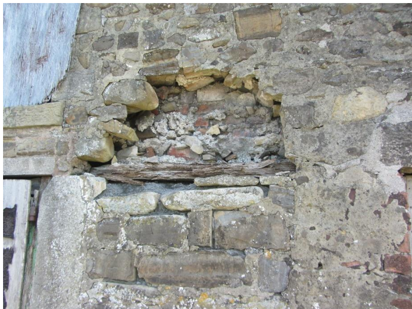
Photo 18 – Front wall missing stones
