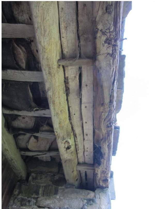
Photo 20 – Rear wall – decayed lintel
