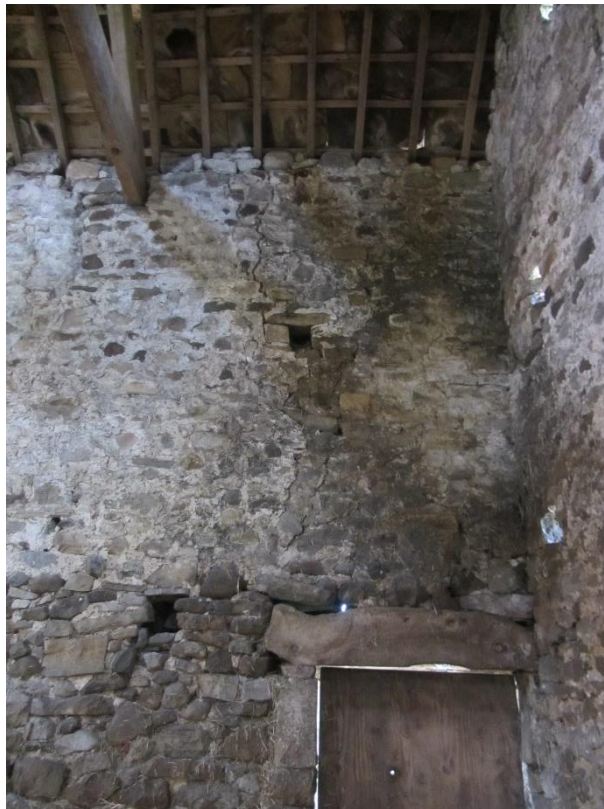
Photo 14 – Vertical cracking – north west corner
