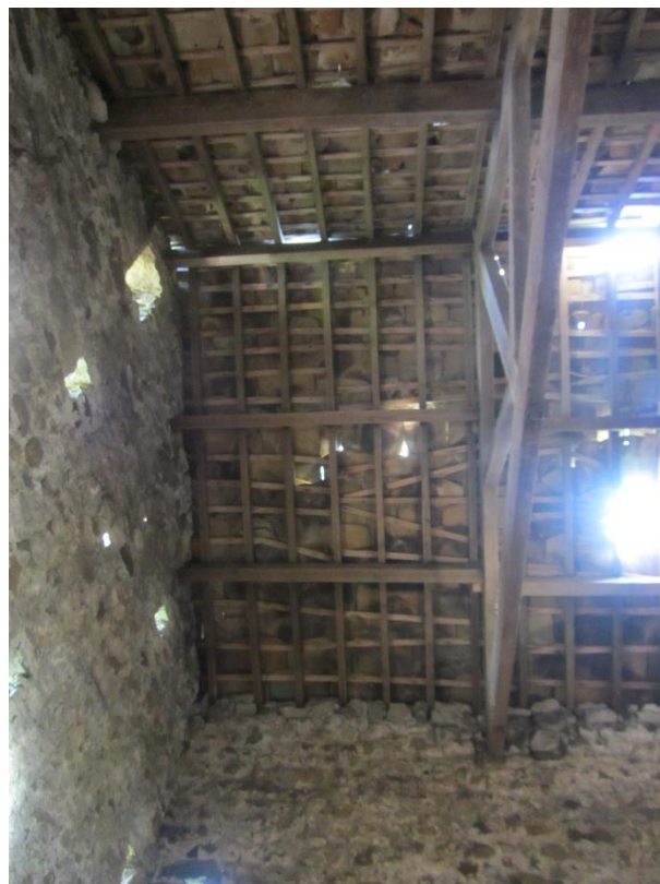
Photo 8 – Slipped slates and battens
