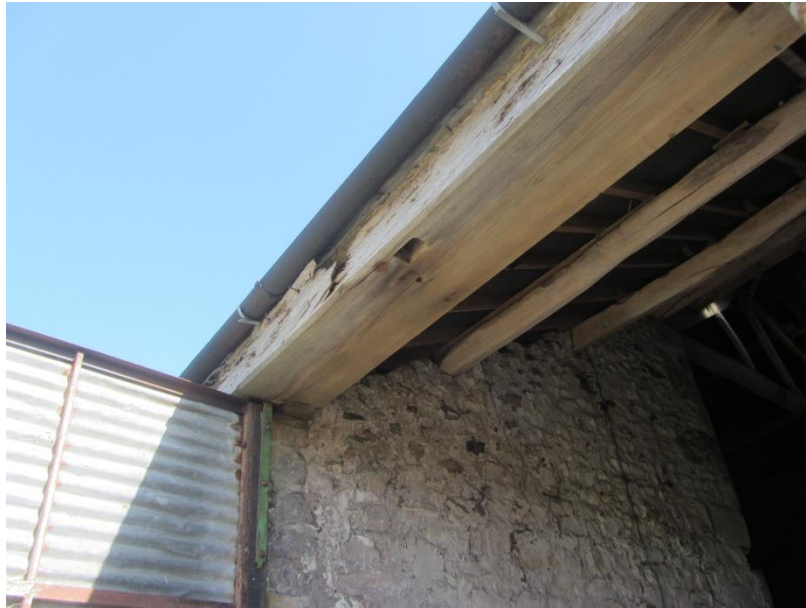
Photo 17 – Front wall – decayed lintel
