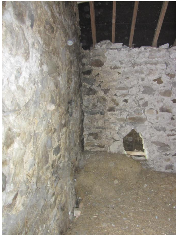
Photo 16 – Vertical cracking and separation
