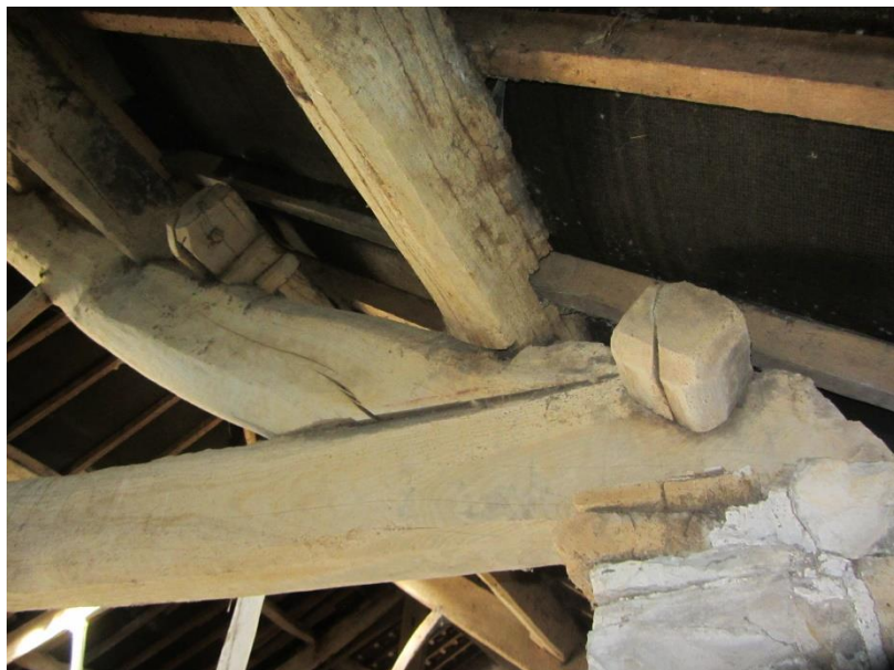
Photo 12 – Decayed roof truss
