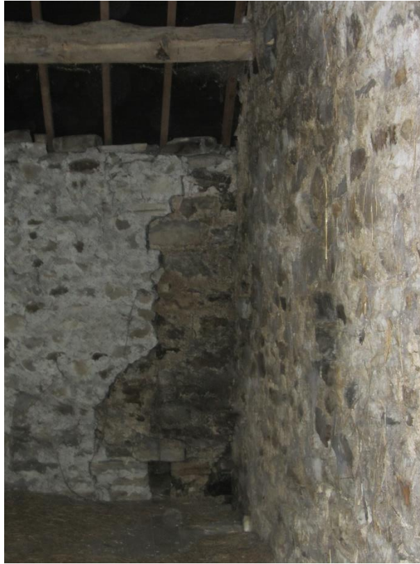
Photo 15 –Vertical cracking – south east corner
