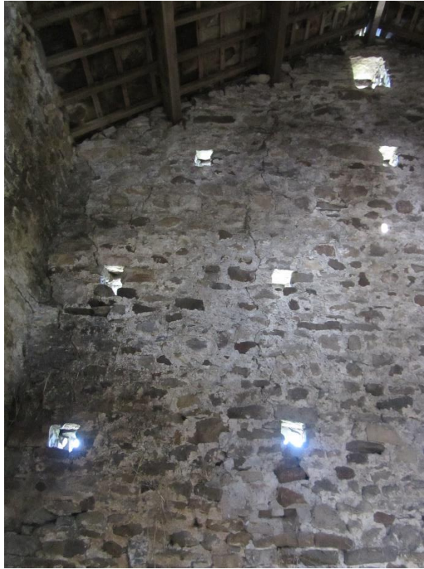
Photo 13 – Vertical cracking – north west gable wall
