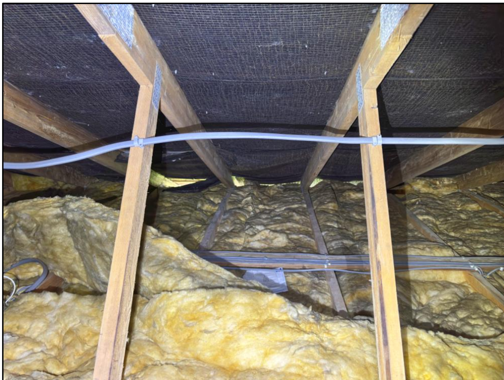
Image of roof void showing layers of rock wool as well as light spillage along the roof edge due to missing soffits, June 2026.
