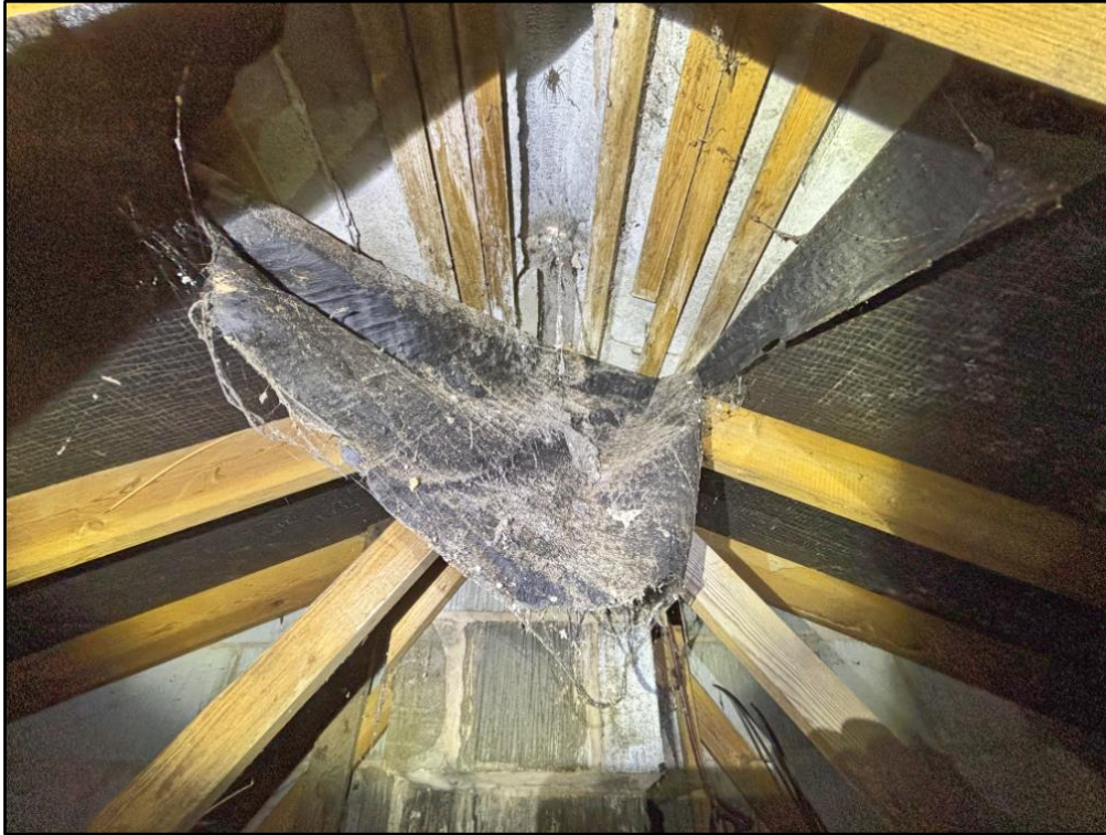
Image of roof void showing sagging and torn roof liner, June 2026.
