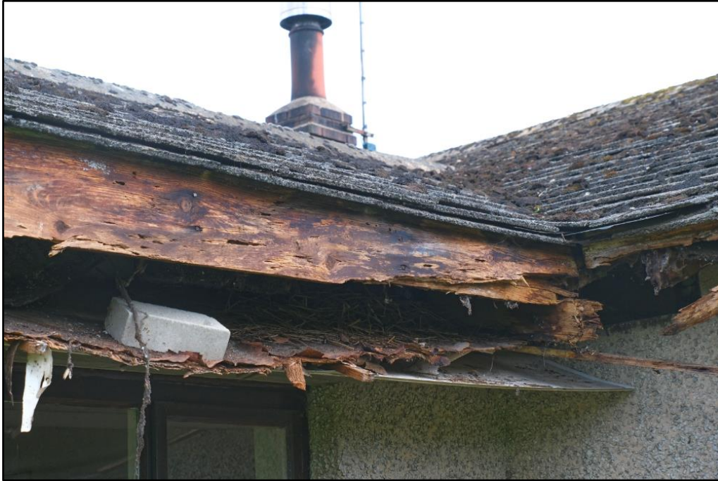
Image showing west (rear) elevation of bungalow with soffits missing June 2026.
