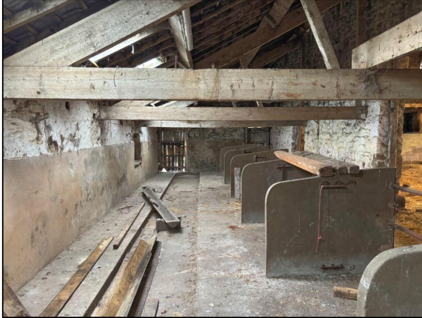
Internal view of Shippon showing light conditions due to presence of roof lights
