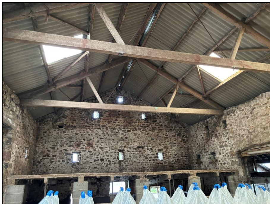
Internal view of haybarn showing roof underside and wall vents (eye holes)
