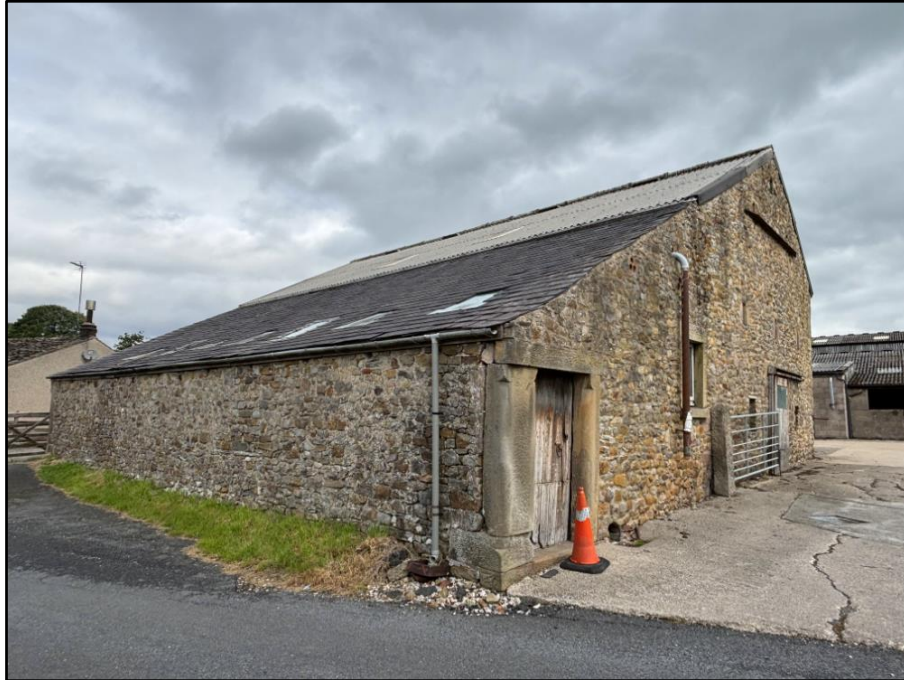
Image of barn (B2) showing south east (farm entrance) and south west (roadside) elevations
