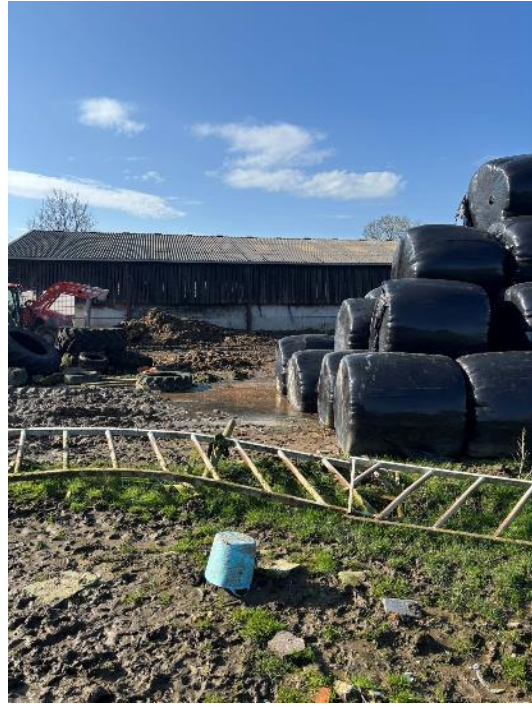
Photograph 3: Overview of the location of the new building. Formerly sheep grazed pasture.
