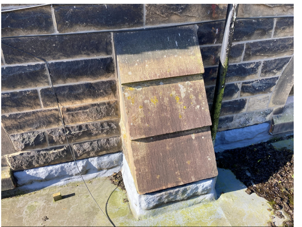
Photo 3: Showing existing surface faced upstand which is resulting in water ingress (roof 2)
