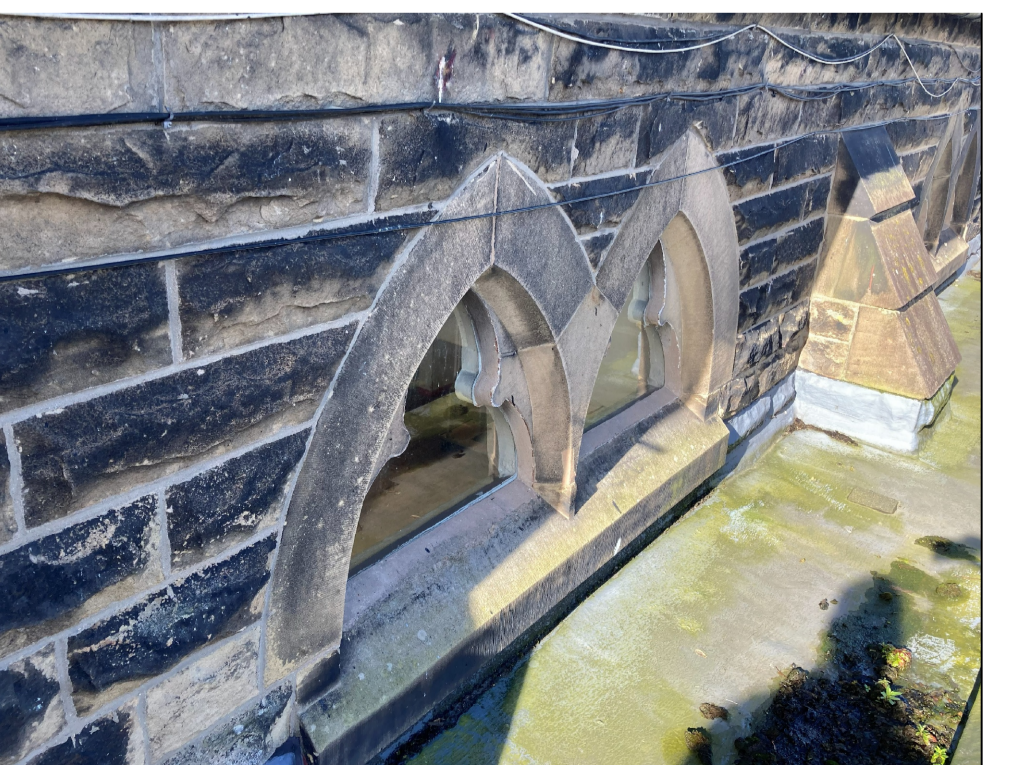
Photo 4: Showing existing stone window reveal with very low upstand beneath which is resulting in water ingress (roof 2)
