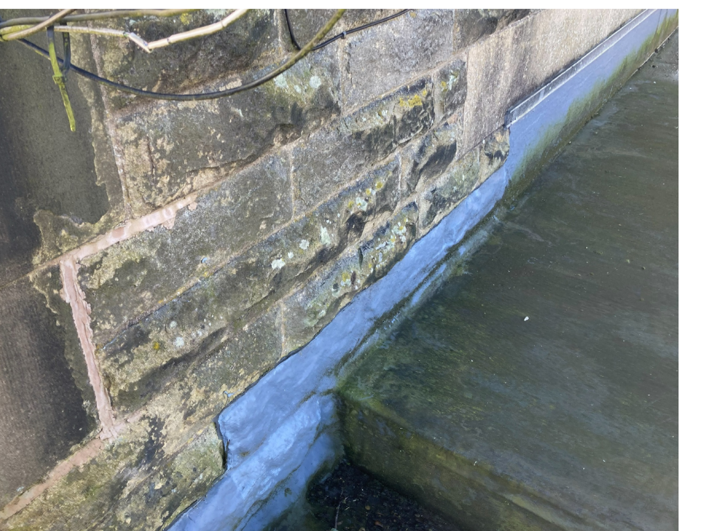
Photo 5: Showing existing surface faced upstand which is resulting in water ingress (roof 1)
