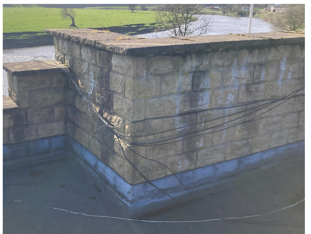
Photo 2: Showing existing surface faced upstanding which is resulting in water ingress (roof 2)
