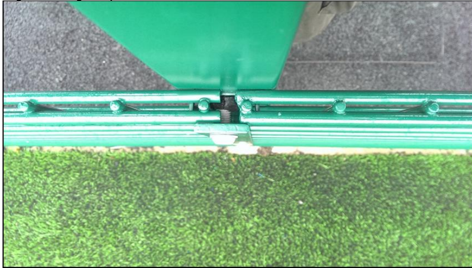
Figure 8: Image showing neoprene isolators
