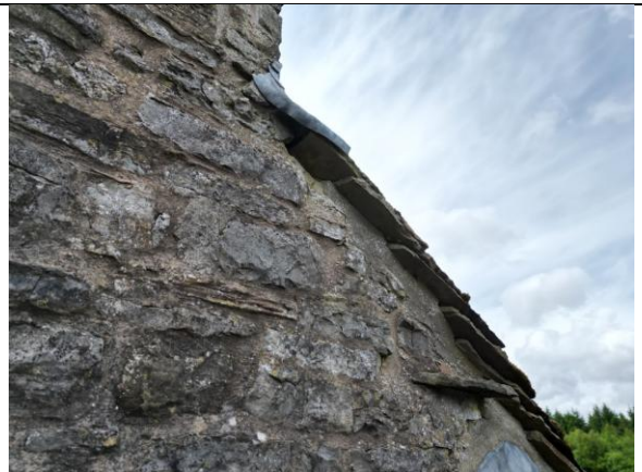
Photograph 12: Gap in western gable
