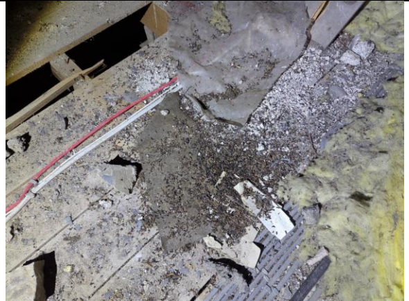
Photograph 20: Pile of droppings in eastern end
