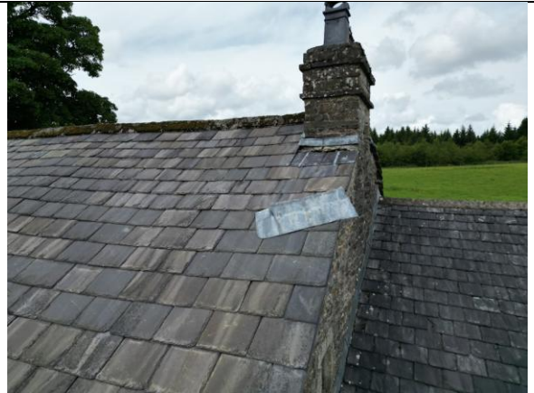
Photograph 10: Damaged chimney flashing
