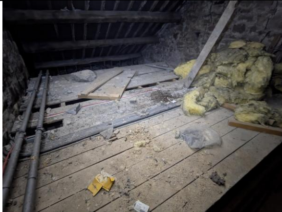
Photograph 19: Boarding in eastern side
