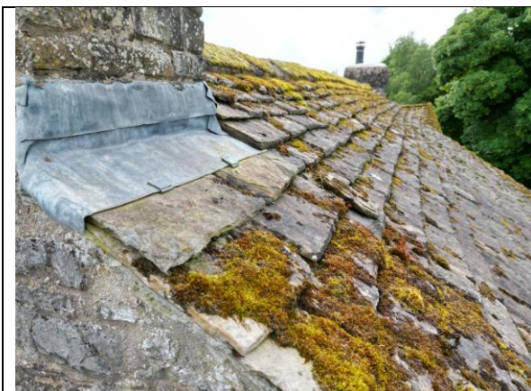
Photograph 13: Western chimney flashing
