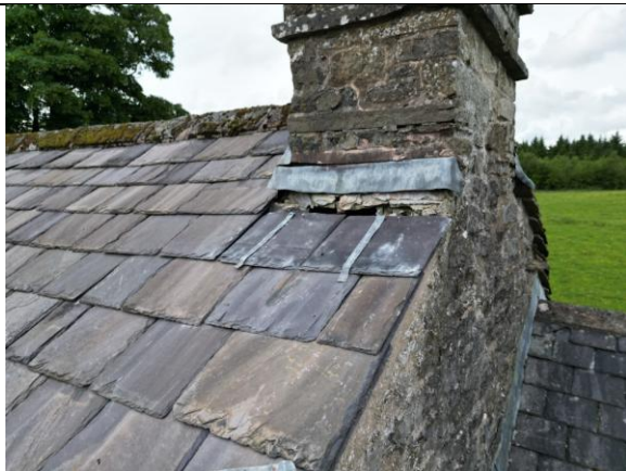
Photograph 11: Damaged chimney flashing
