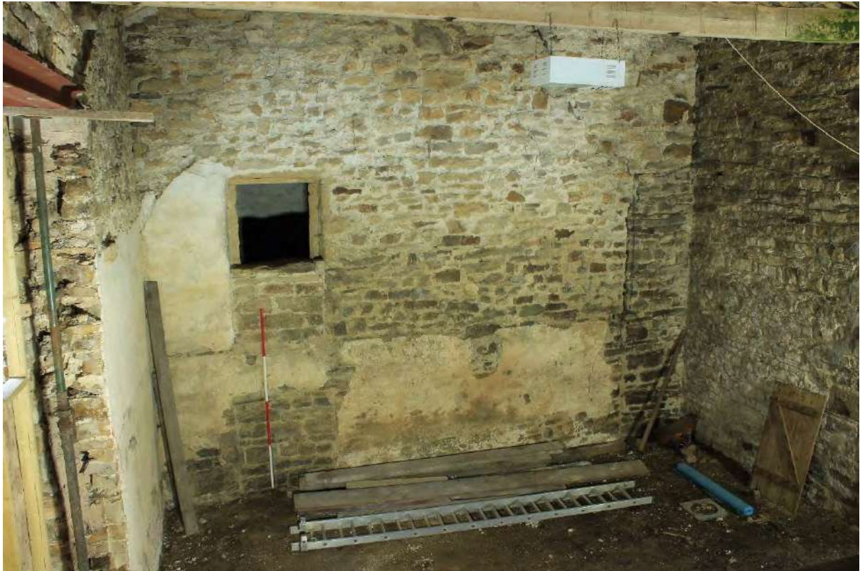
Plate 27b North (left), east (centre) and south (right) walls of Bay 3 in Building A, looking east
