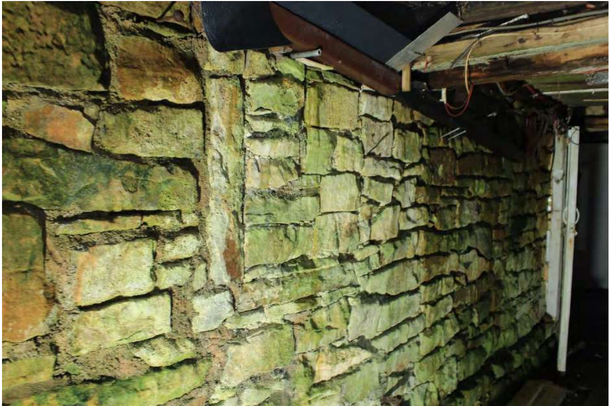
Plate 35b was 35 Stone wall (Wall D) to the south of Building B, looking south-west
