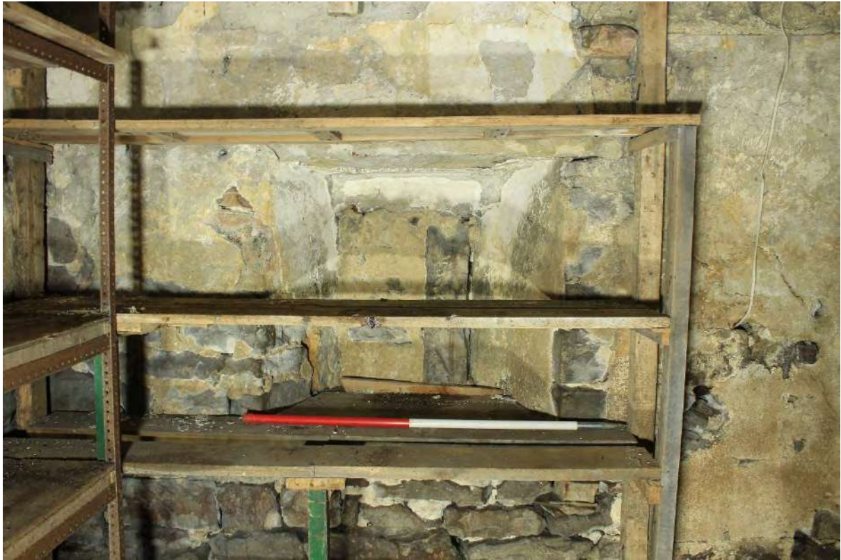
Plate 32d Blocked opening in the north wall of Bay 4 of Building A
