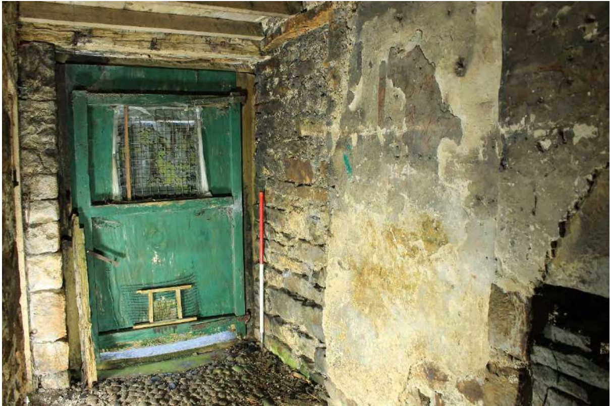
Plate 32b South (left) and west (right) walls of Bay 4 of Building A
