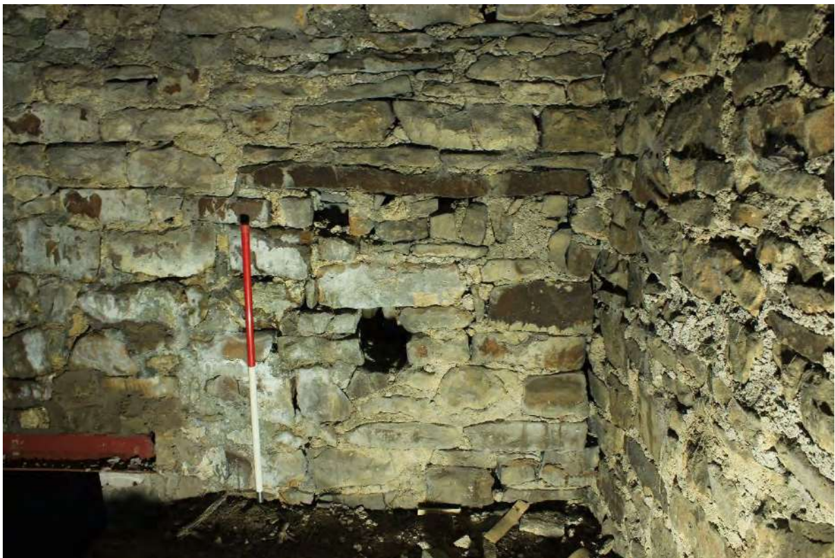
Plate 33a West (centre) and north (right) walls of the first-floor hay loft in Bay 1 of Building A, looking west
