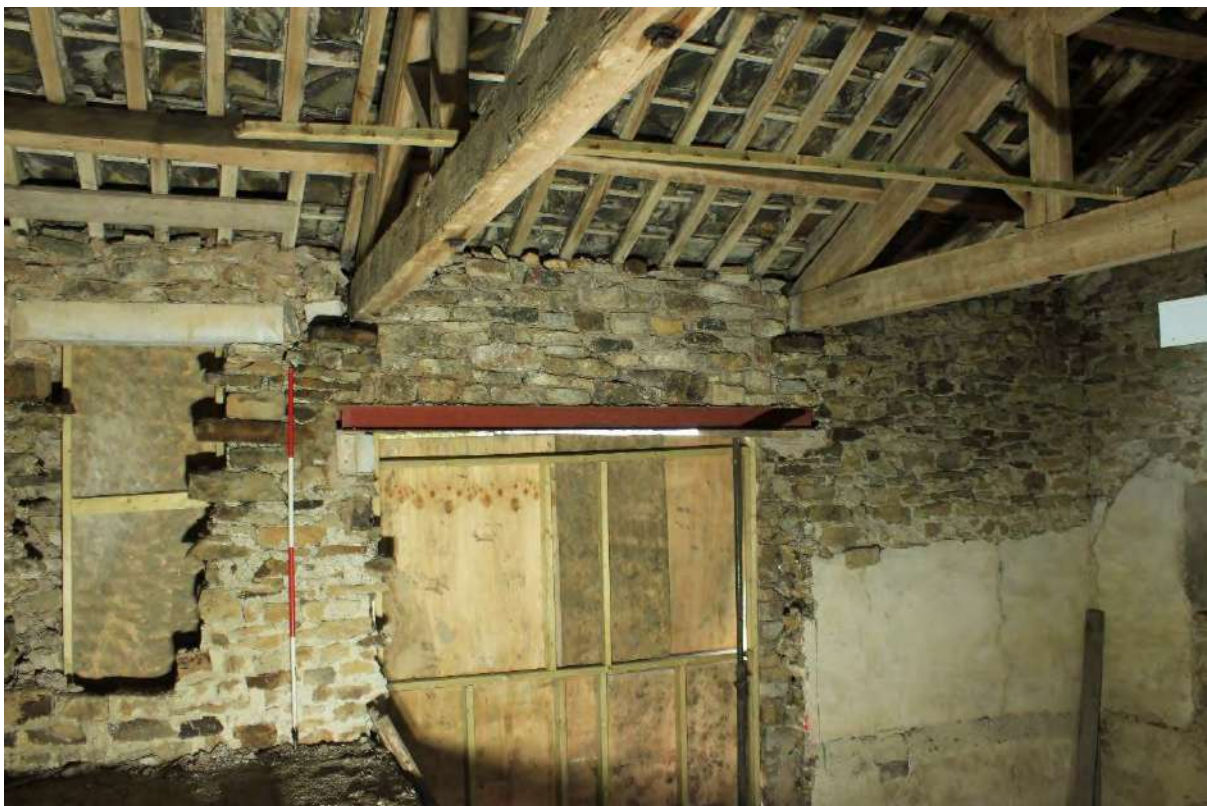
Plate 44 North wall of Building A at first floor level with pitching loft opening (left) and north wagon doorway (centre), looking north
