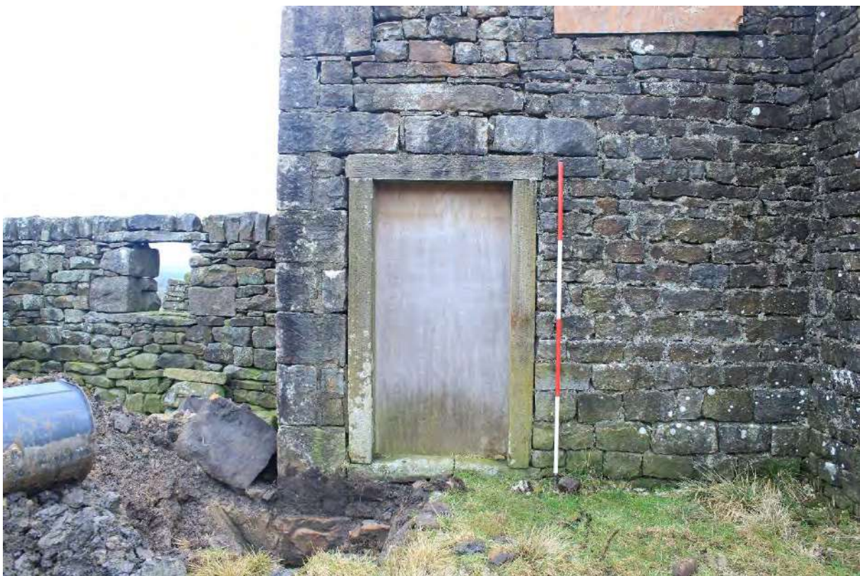
Plate 20 Boarded up doorway opening at the west end of the south elevation
