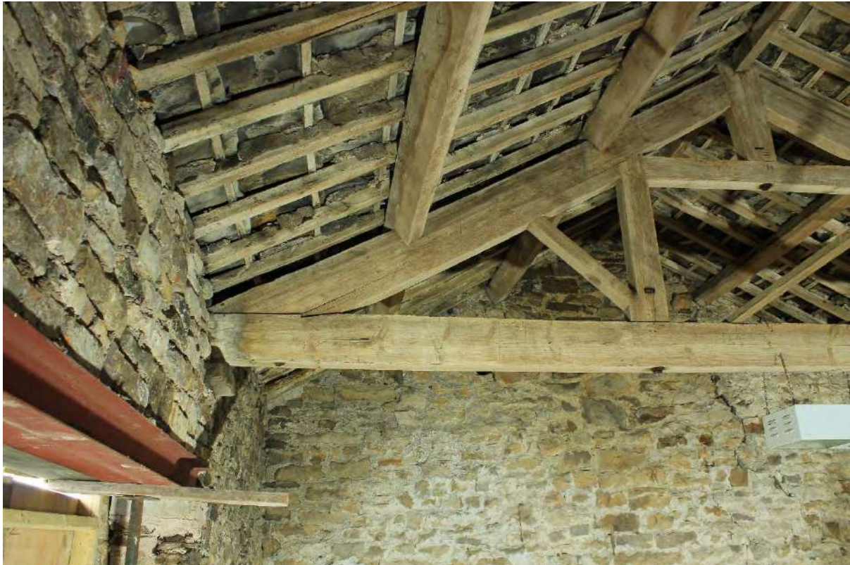
Plate 45 North wagon doorway (left) east roof truss in Building A, looking east
