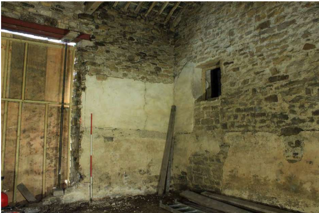
Plate 27a Boarded north wagon doorway (left), north (centre) and east (right) walls of Bay 3 in Building A, looking north-east
