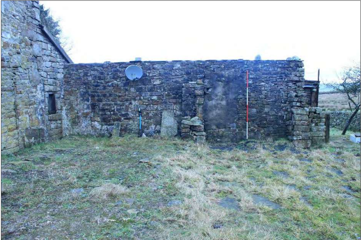
Plate 11 South elevation of Walls D and E to the south of Building B, looking north
