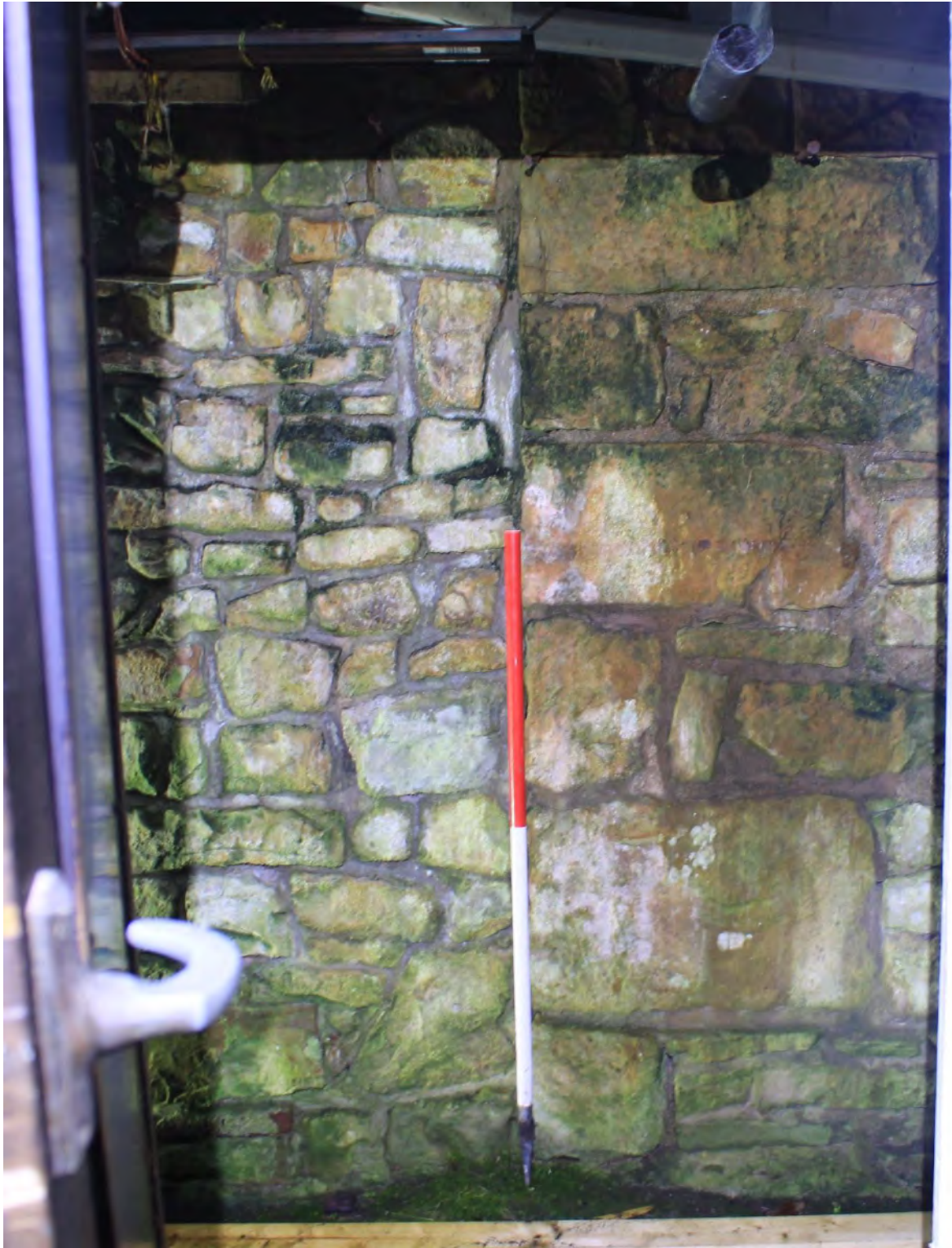
Plate 35a Straight joint in stone wall to the south of Building B marking north-east corner (quoins) of former building (Wall D right) and Wall E (left), looking south from the kitchen in Building B
