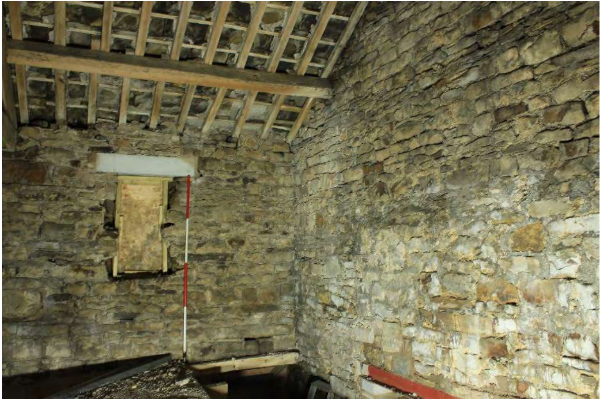
Plate 34 South wall of the loft over the byre, showing boarded pitching opening
