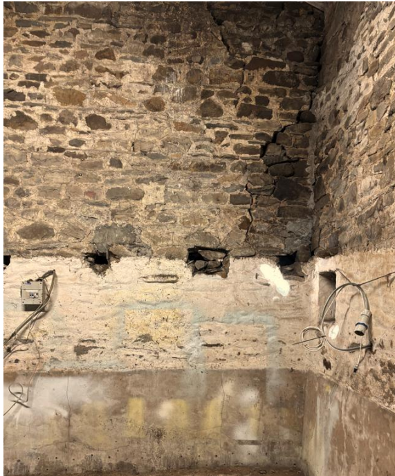
Photograph (3) – Showing crack that requires crack stitching
