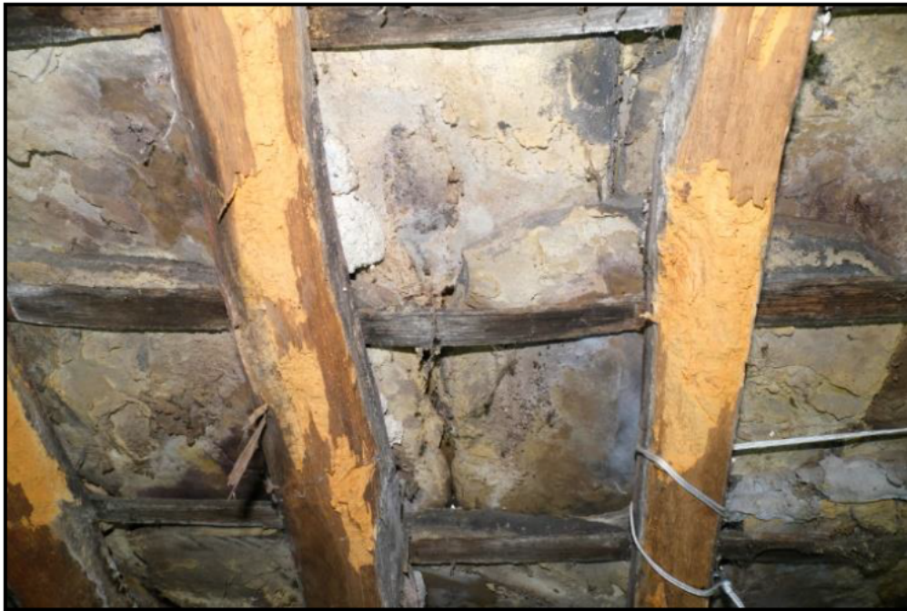
Image showing close up of roof underside, no liner and worn roof timbers.
