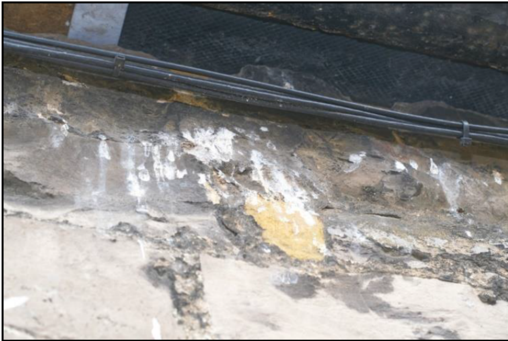
Image showing bird droppings below roof edge located at 55 Downham Road (immediate adjacent 57 Downham Road). A starling was seen entering this location during the survey.
