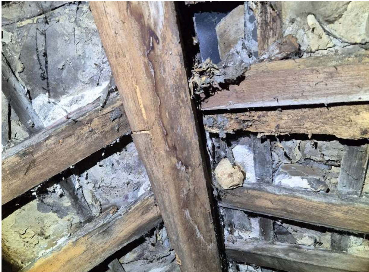
Figure 1: Failed ridge beam.
