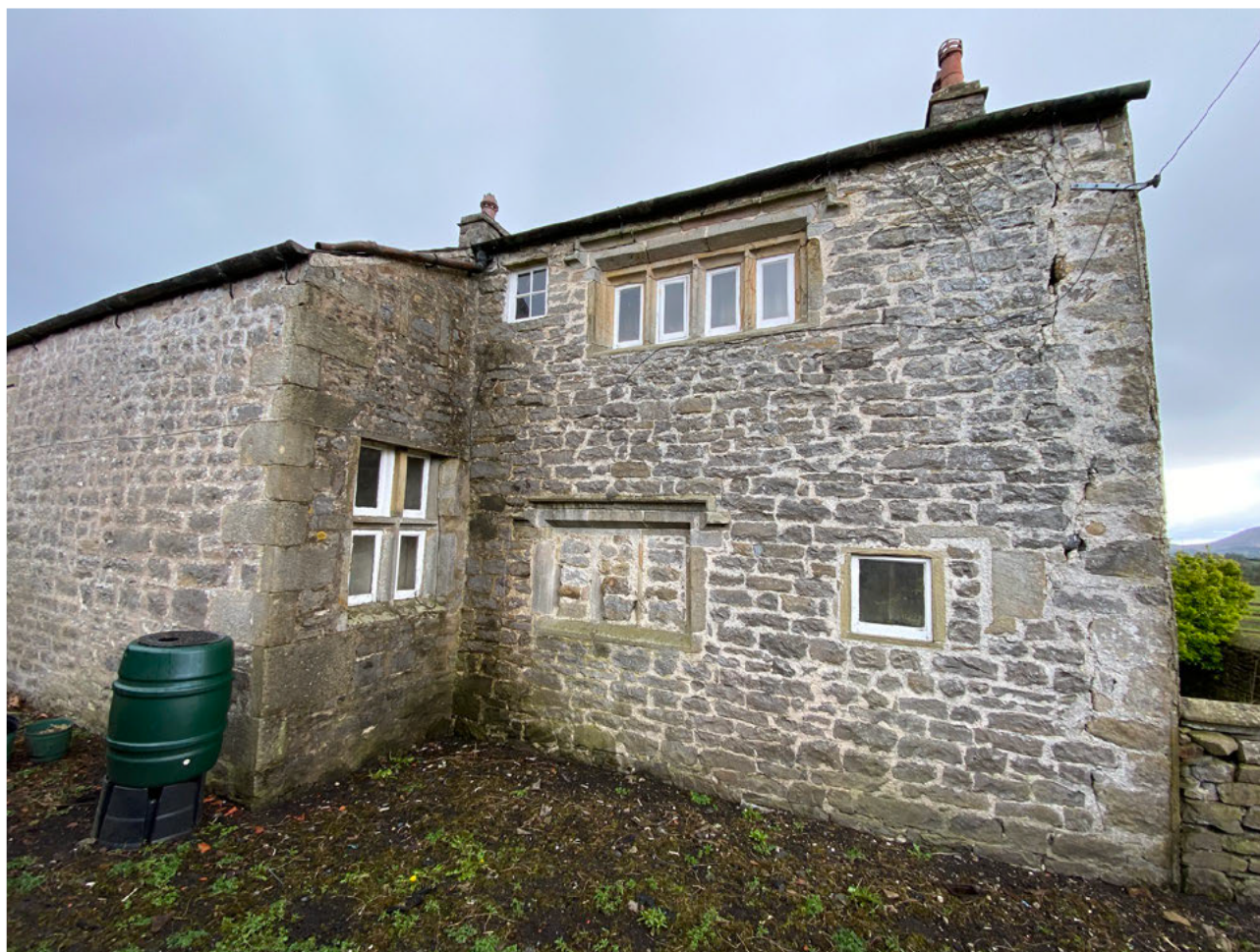
Plate 8 - Rear elevation from the north west corner, evidence of changes to fenestration.
