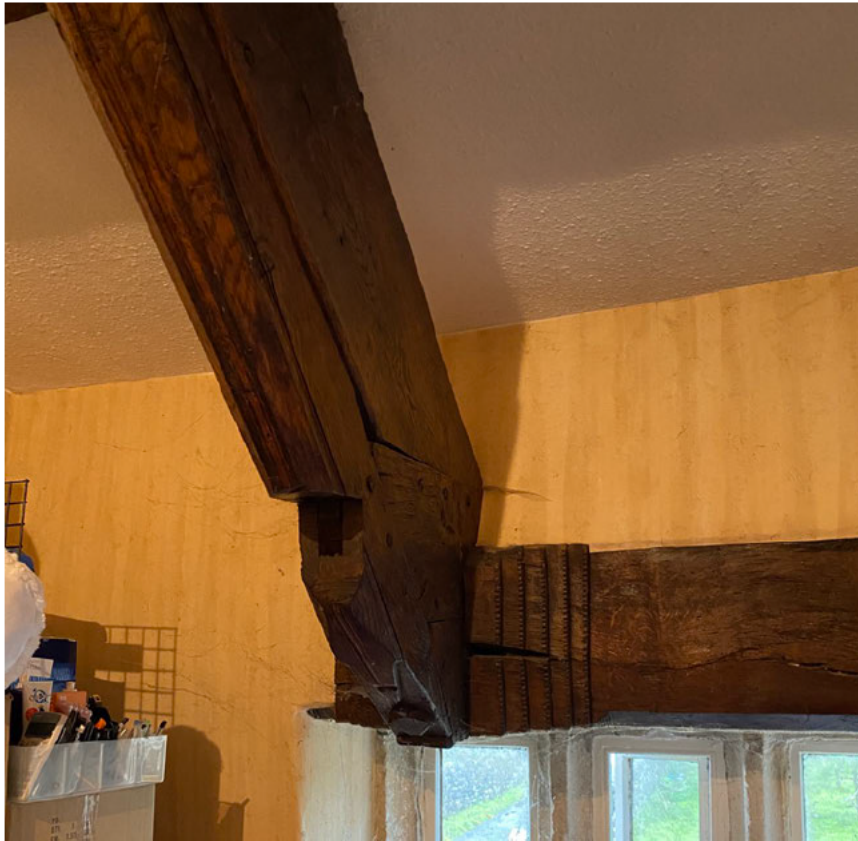
Plate 13 - Truss has been cut to accommodate window
