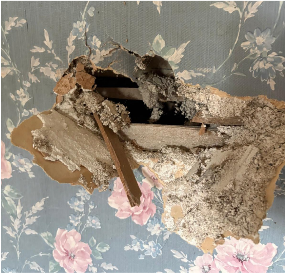
Plate 10 - Internal partition wall, opened up to reveal 19th century lath and plaster wall
