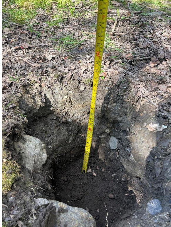
Image 1. Trial hole, showing nom. 200mm thickness of topsoil, down to stiff boulder clay.
