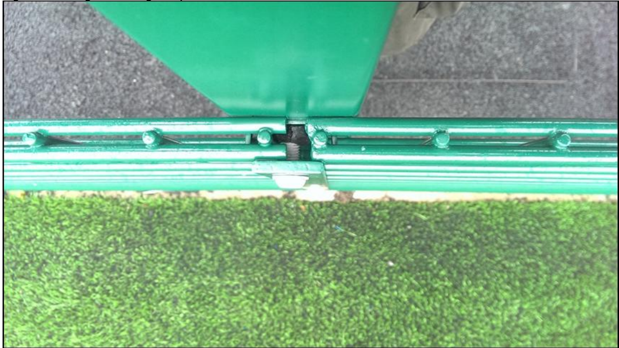
Figure 9: Image showing neoprene isolators
