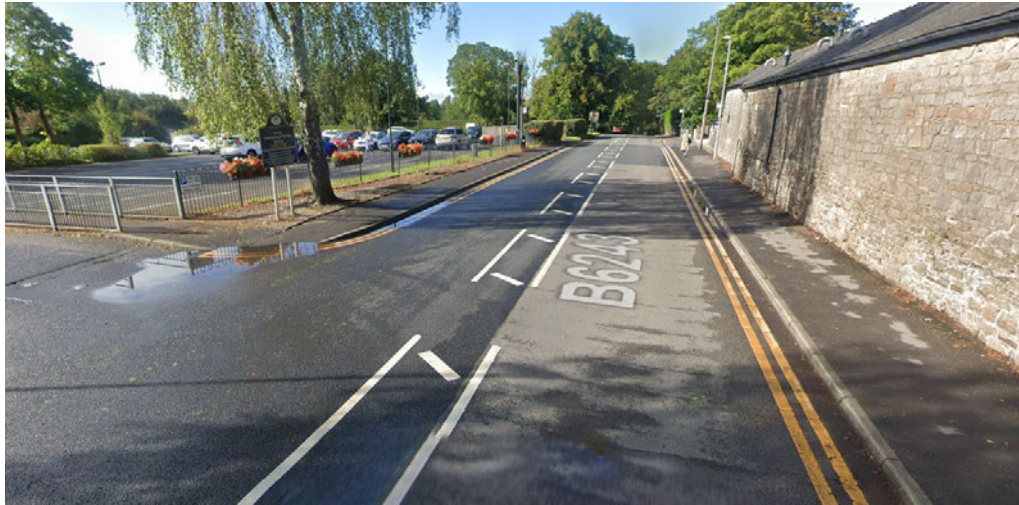
Figure 3.5 Existing carriageway condition and TROs (Edisford Road) Source: Google Maps, obtained 12/02/2026
