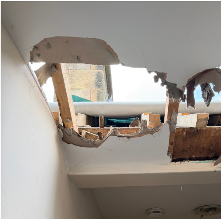
Image 8 Valley Gutter (internal damage)
