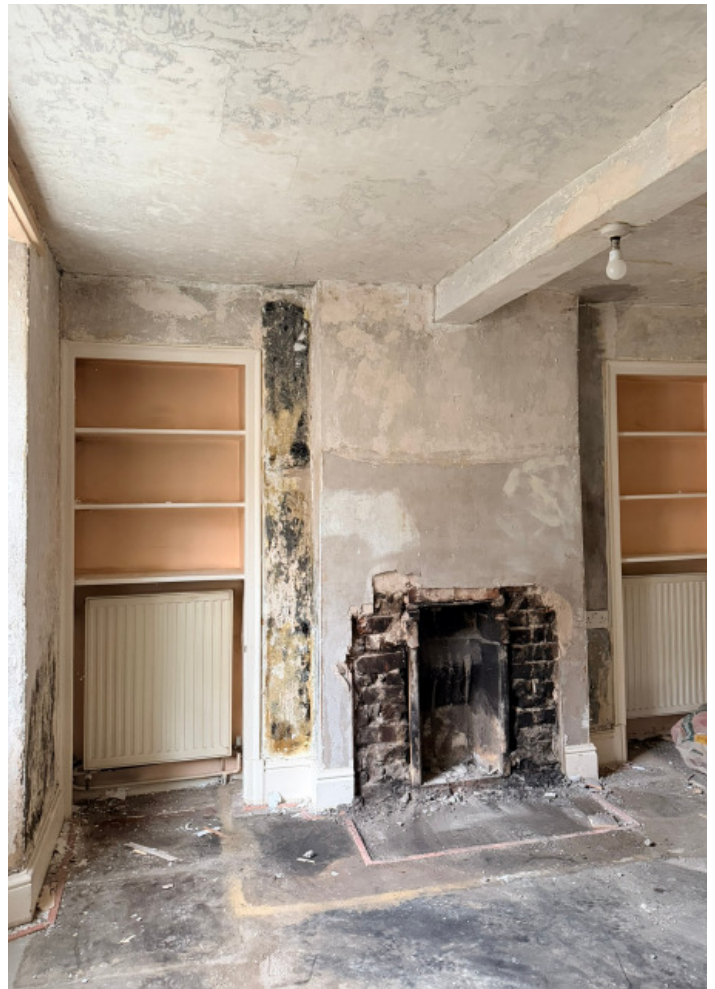
Image 11 Existing radiators (lounge)
