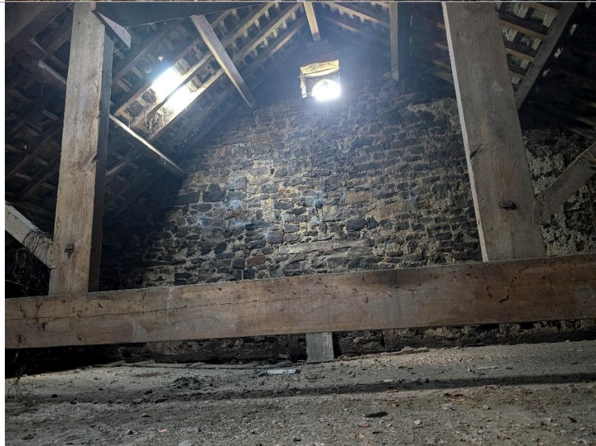
Photo 10. Loft of workshop (former stables) with circular window aperture (main roost egress point).
