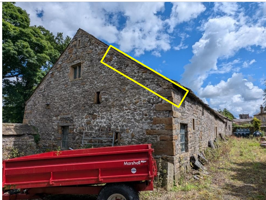
Photo 4. South-west elevation (several gaps in stonework).
