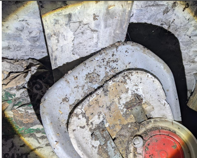
Photos 3.3a & 3.3b Droppings and feeding remains within upper floor of central section.
