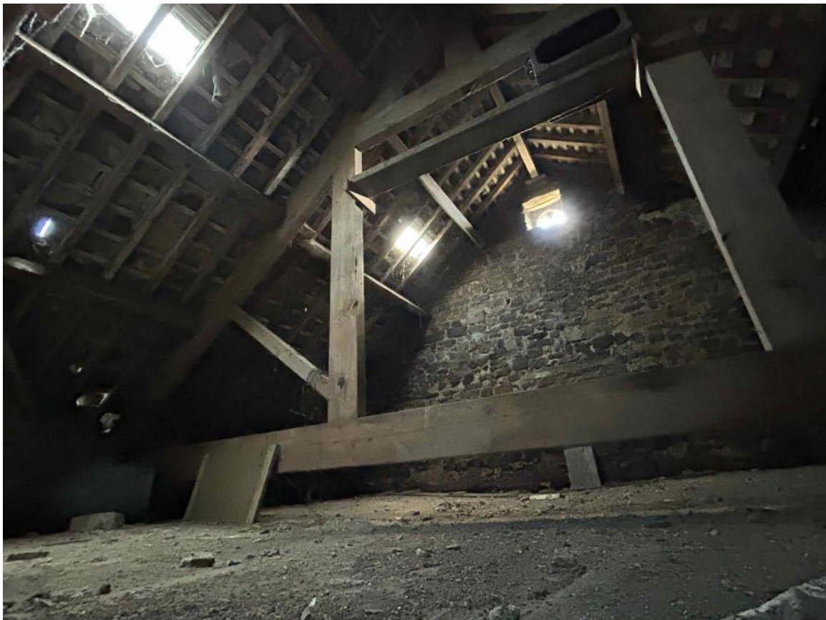
Photo 14: Queen Post Truss Over Workshop (Note: Only 300mm Between Tie Beam & Floor Level)
