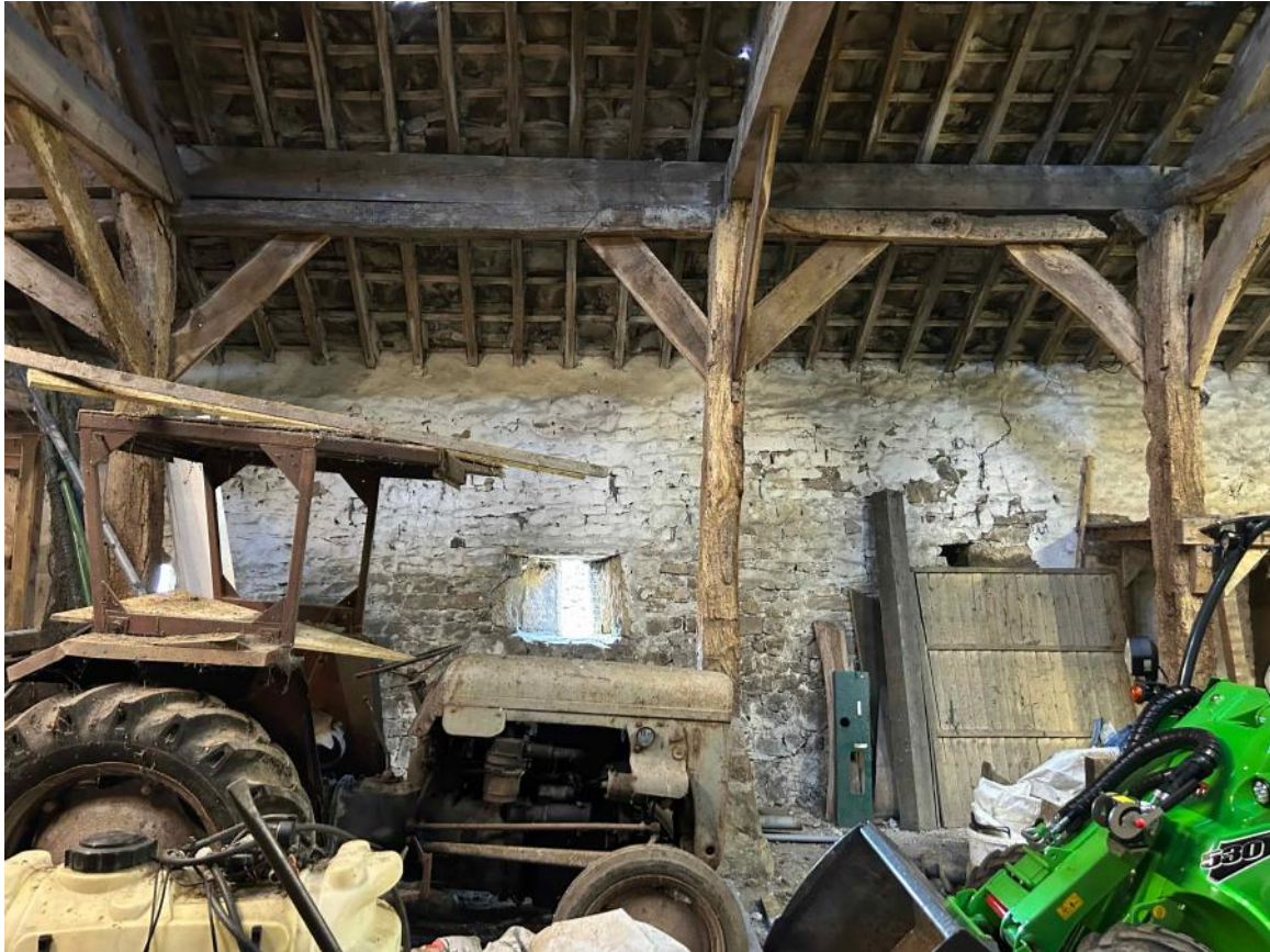
Photo 11: Bays 5 & 6 (South) - Lower Purlin Not Connected
