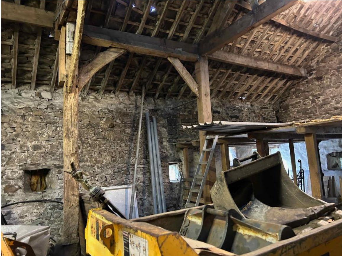
Photo 7: Bay 2 (South) Upper Purlin Not Connected, Lower Twisted & Braces Pulling Out
