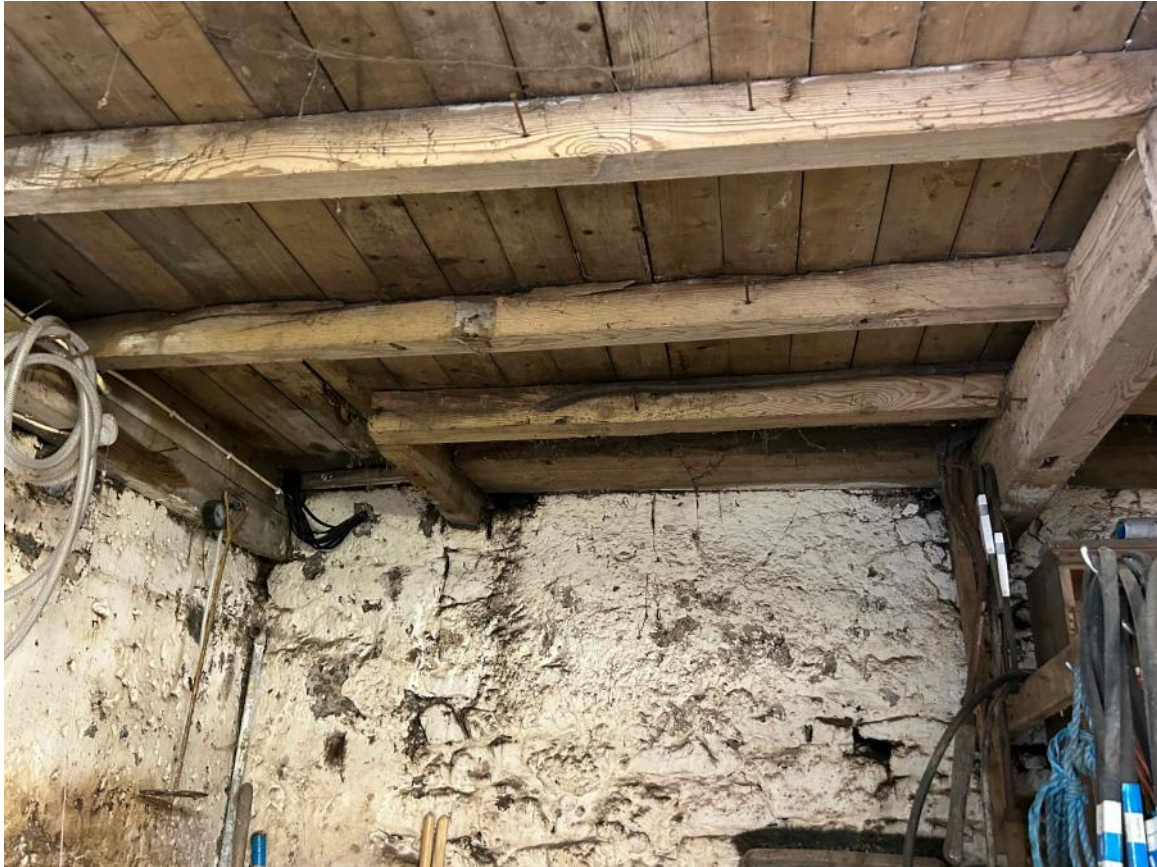
Photo 13: Workshop Joist Split & Inadequately Supported
