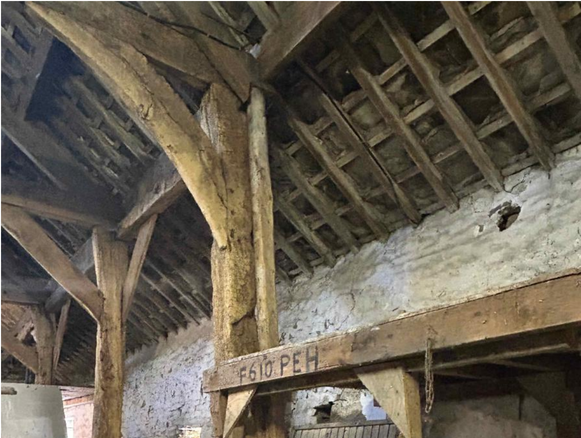
Photo 10: New Rafters Not Adequately Supported
