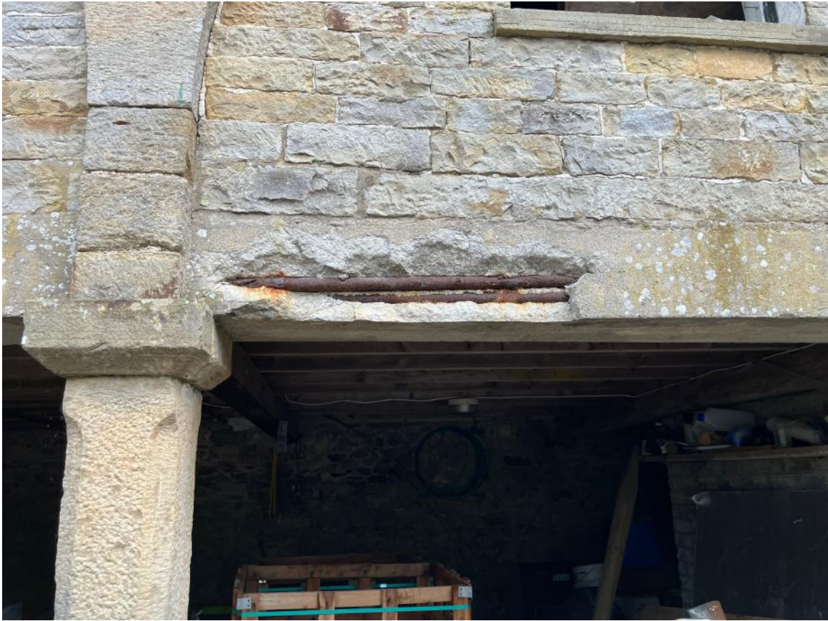
Photo 16: Spalled Concrete Lintel - Reinforcement Exposed & Corroding
