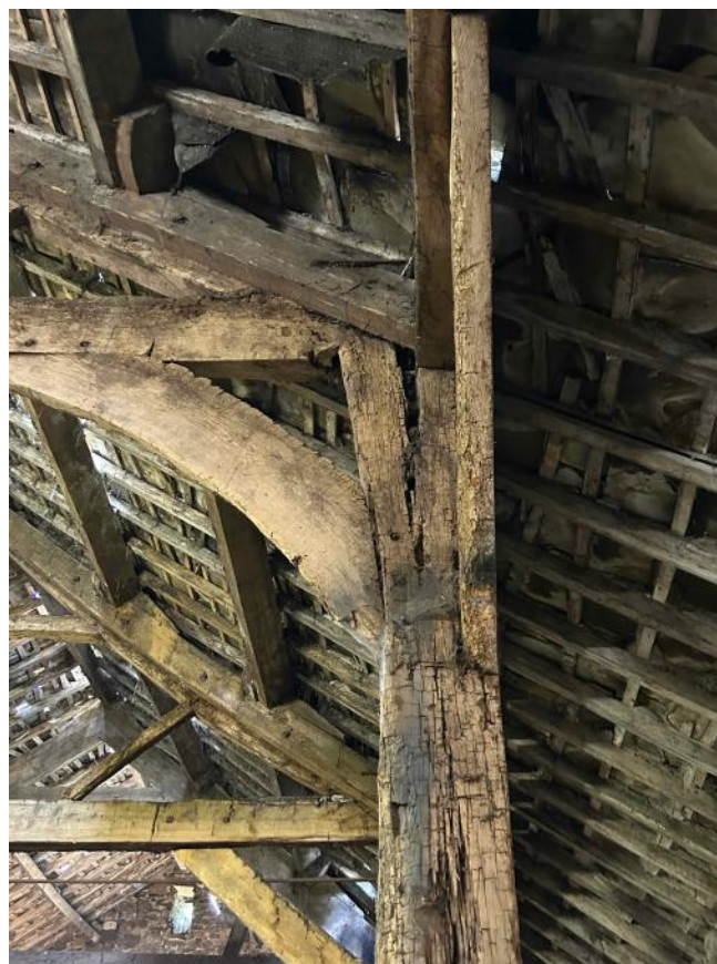
Photo 8: Frame No.3 - Split in Post
