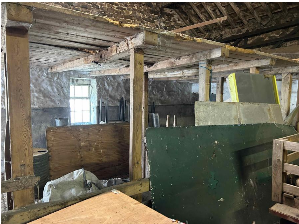
Photo 12: Existing Mezzanine Structure Inadequate for Access
