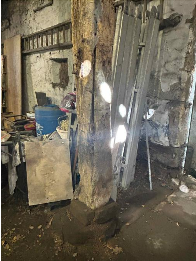
Photo 9: Frame No.3 - Vertical Shake in Post
