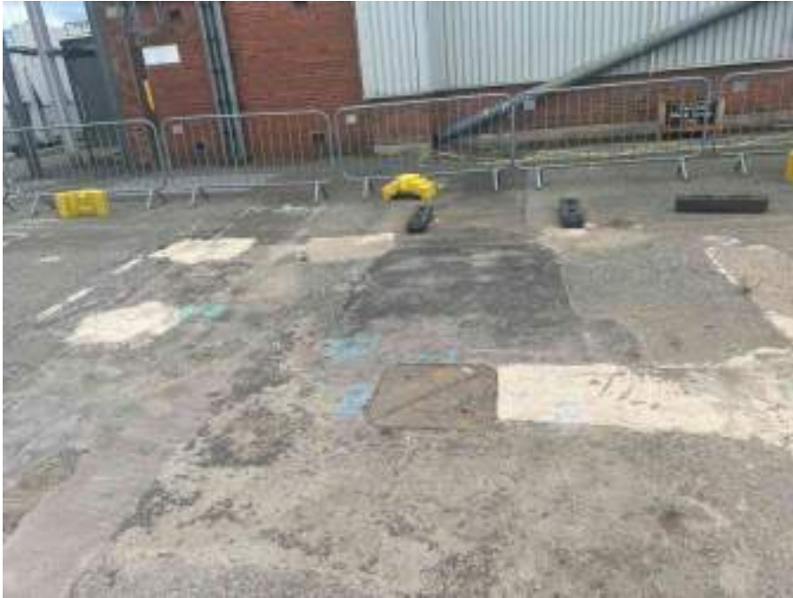
MH07X_U_14082025_1229_053.jpg, 00:00:00, 0.00 m Start node, manhole, reference: MH08, MANHOLE LOCATED ADJACENT TO LOADING BAY
