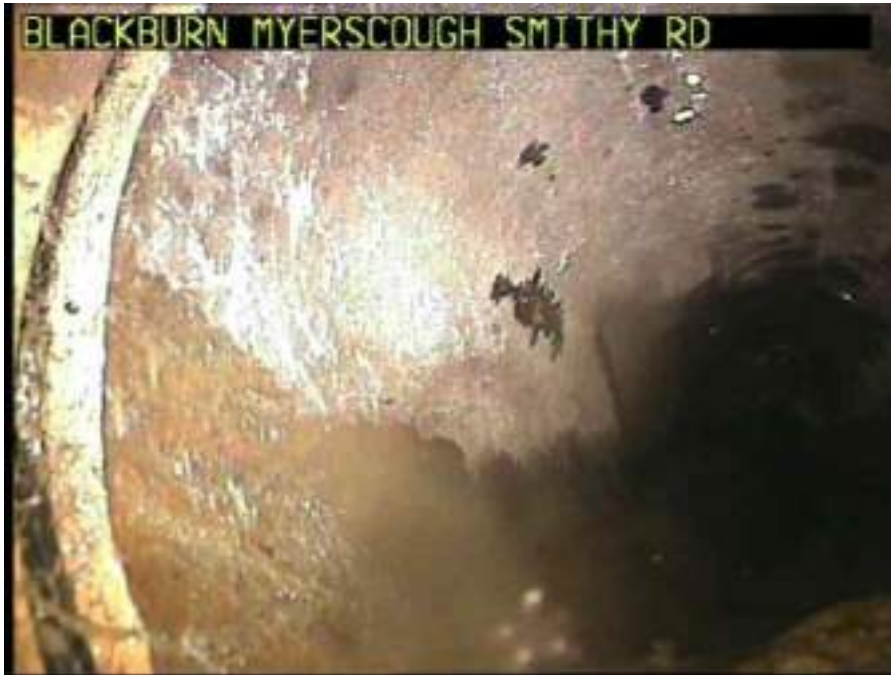
MH02X_D_13082025_1042_023.jpg, 00:00:41, 1.60 m Settled deposits, coarse, 10% cross-sectional area loss
