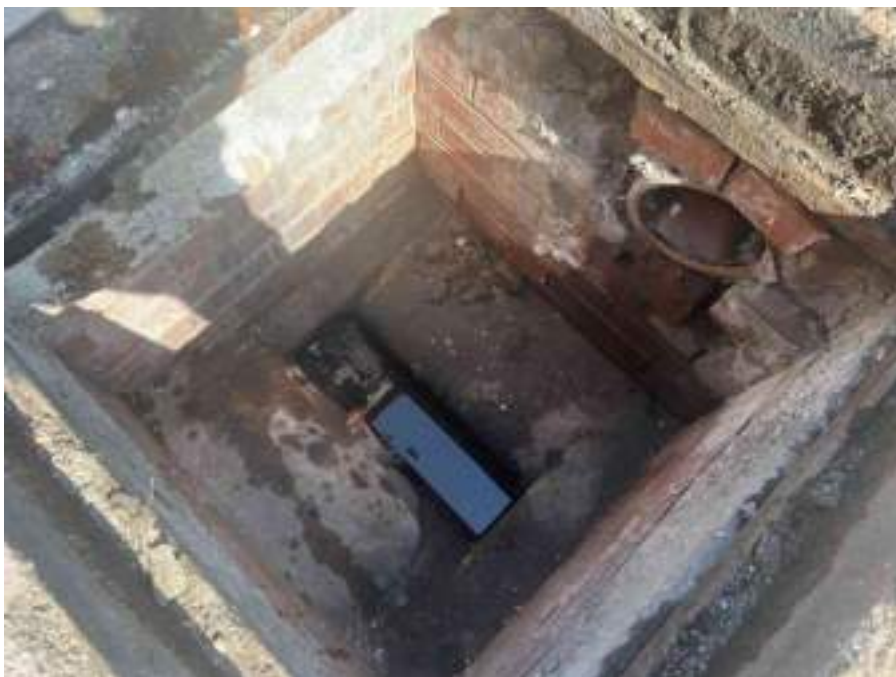
MH02X_D_13082025_1042_022.jpg, 00:00:00, 0.00 m Start node, manhole, reference: MH02, MANHOLE LOCATED ADJACENT TO STAIRCASE
