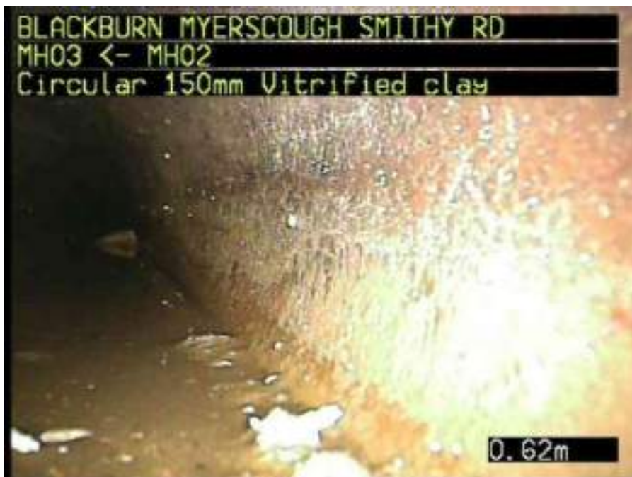
MH03X_U_13082025_1034_016.jpg, 00:00:21, 0.62 m Settled deposits, coarse, 5% cross-sectional area loss, start
