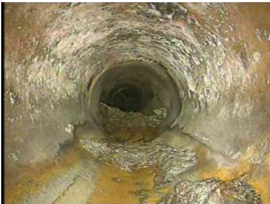
MH08AX_U_14082025_1232_070.jpg, 00:05:07, 39.43 m Settled deposits, coarse, 5% cross-sectional area loss
