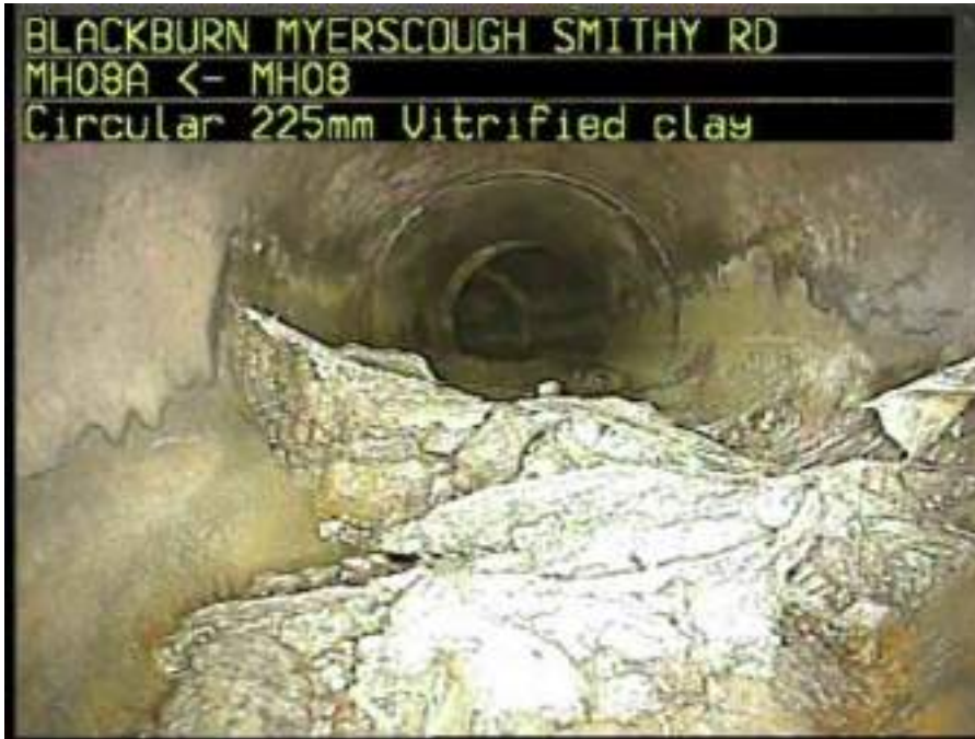
MH08AX_U_14082025_1232_071.jpg, 00:05:14, 40.22 m Settled deposits, coarse, 30% cross-sectional area loss
