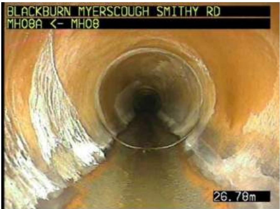
MH08AX_U_14082025_1232_068.jpg, 00:02:36, 26.78 m Attached deposits, encrustation from 9 o'clock to 11 o'clock, 5% cross-sectional area loss
