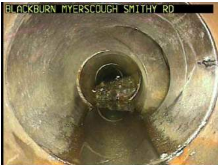
MH07X_U_14082025_1229_056.jpg, 00:00:15, 0.70 m Fracture, longitudinal at joint at 2 o'clock
