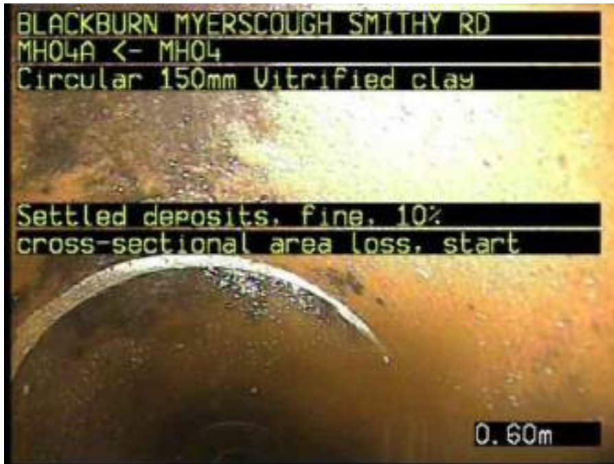
MH04AX_U_13082025_1217_041.jpg, 00:00:04, 0.60 m Settled deposits, fine, 10% cross-sectional area loss, start
