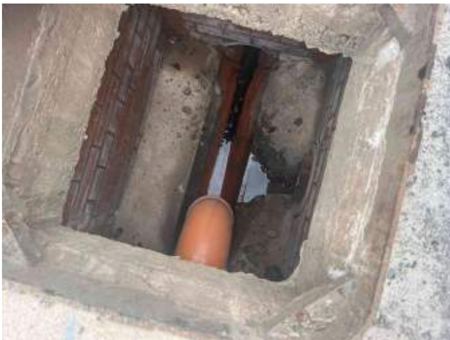
MH08X_D_14082025_1244_073.jpg, 00:00:00, 0.00 m Start node, manhole, reference: MH08, MANHOLE LOCATED ADJACENT TO LOADING BAY DOOR.
