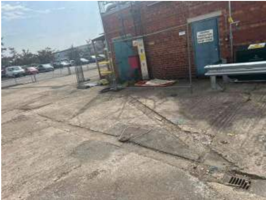
MH04X_D_13082025_1054_031.jpg, 00:01:33, 14.17 m Finish node, manhole, reference: MH05, MANHOLE LOCATED ADJACENT TO FIRE EXIT
