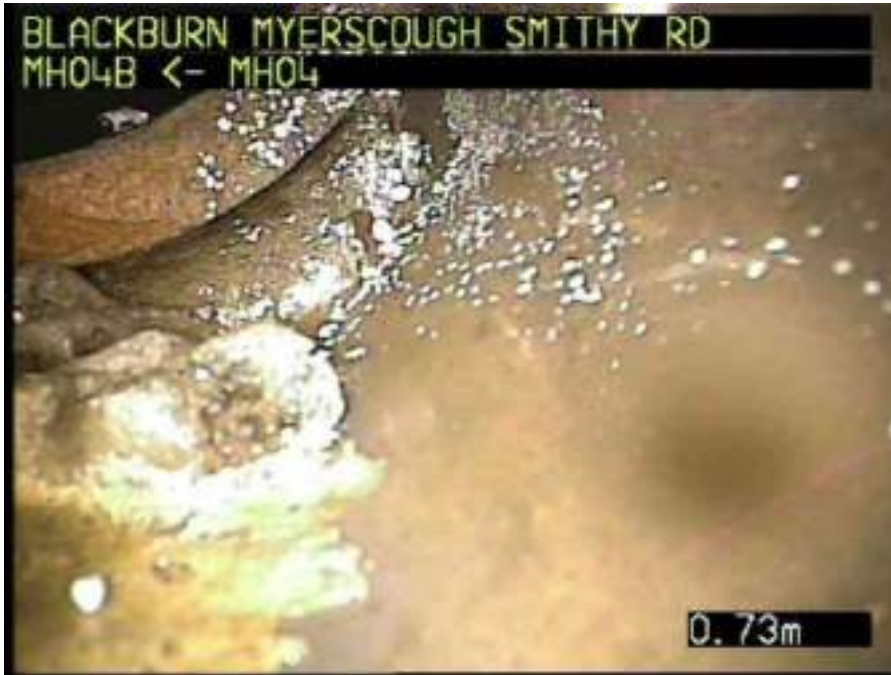
MH04BX_U_13082025_1225_047.jpg, 00:00:08, 0.60 m Joint displaced, large
