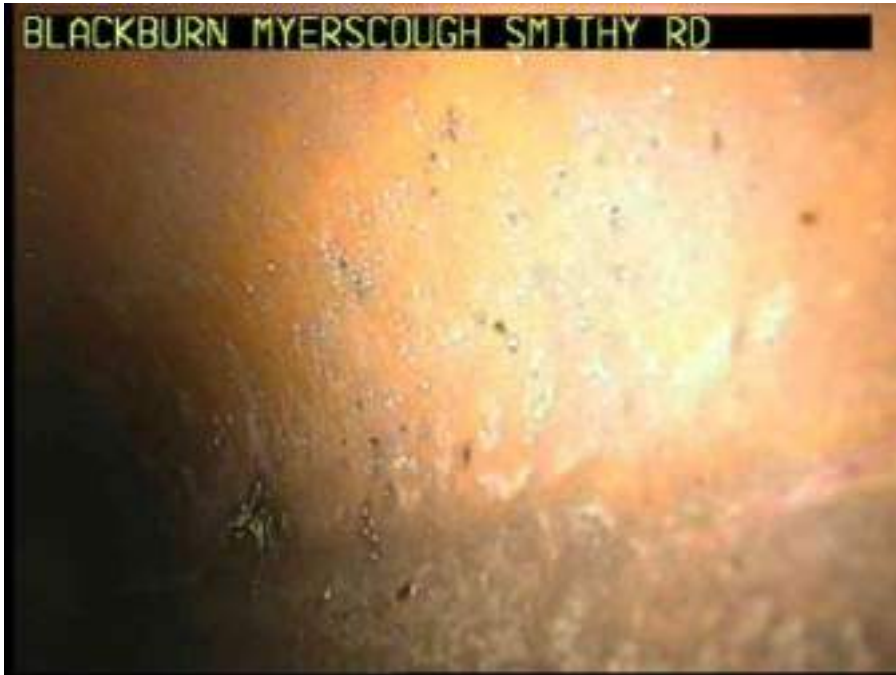
MH09X_D_14082025_1220_050.jpg, 00:00:10, 0.64 m Settled deposits, fine, 10% cross-sectional area loss
