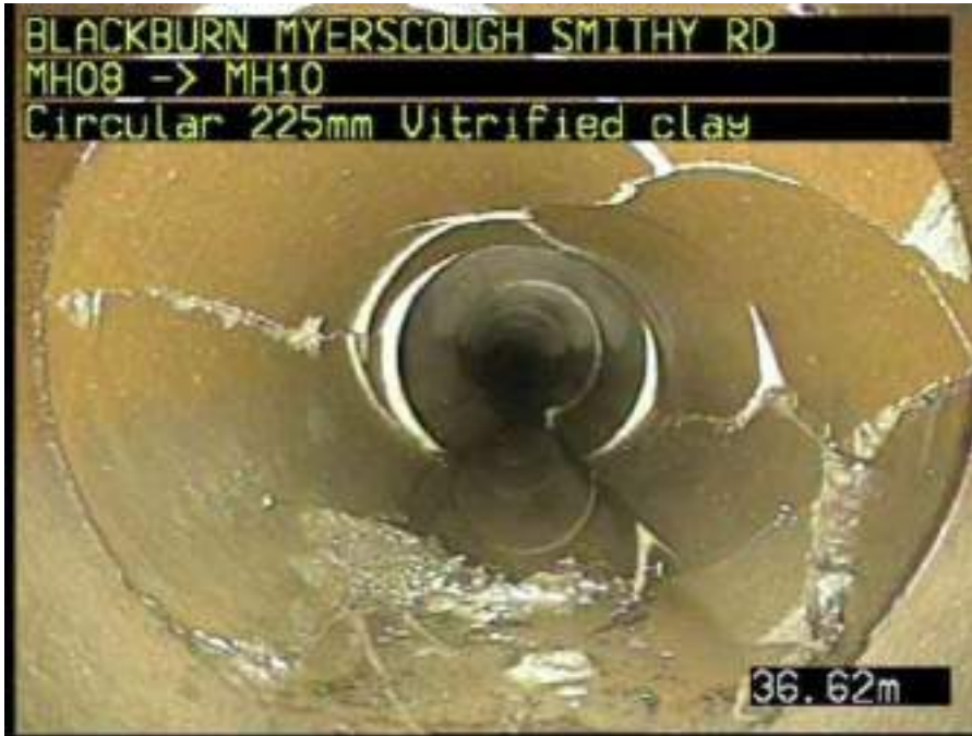
MH08X_D_14082025_1244_084.jpg, 00:06:45, 36.62 m Deformed sewer or drain, 10%
