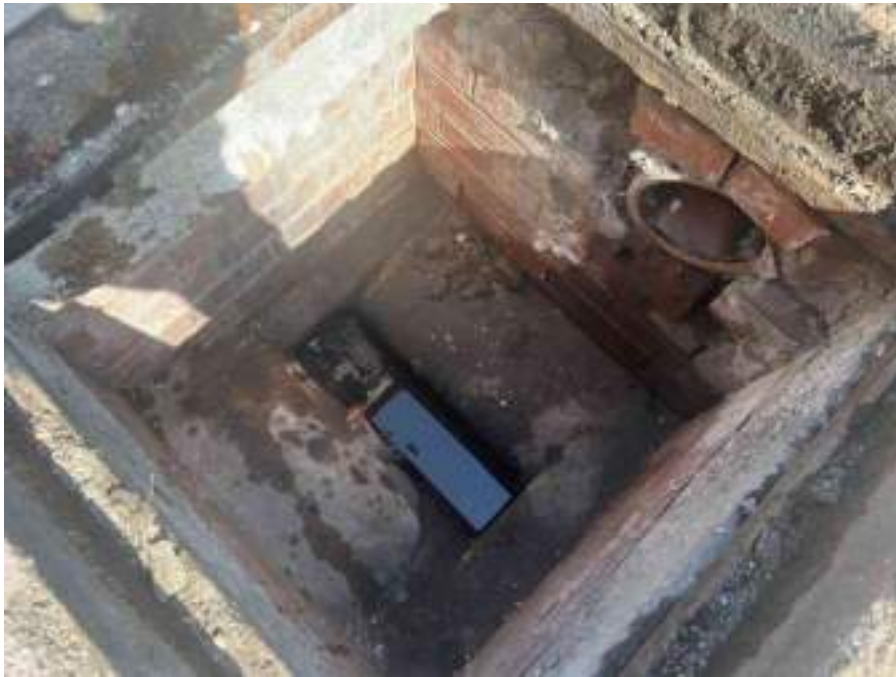
MH01X_D_13082025_0951_005.jpg, 00:00:30, 2.99 m Finish node, manhole, reference: MH02, MANHOLE LOCATED ADJACENT TO STAIRCASE
