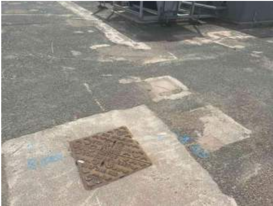
MH07X_D_14082025_1308_058.jpg, 00:00:00, 0.00 m Start node, manhole, reference: MH07, MANHOLE LOCATED ADJACENT TO COOLING STATION
