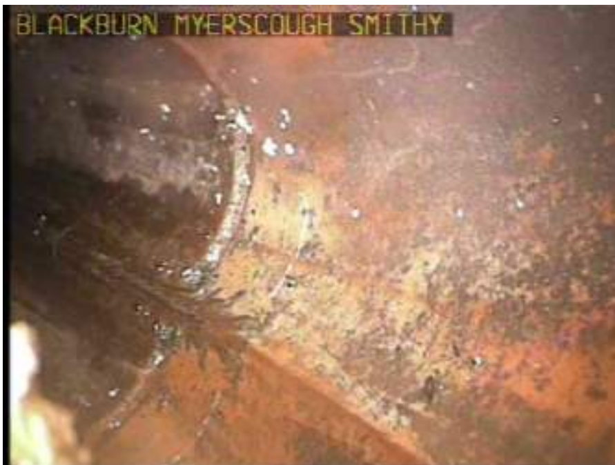
MH03X_U_13082025_1034_018.jpg, 00:01:46, 11.28 m Settled deposits, coarse, 5% cross-sectional area loss, finish
