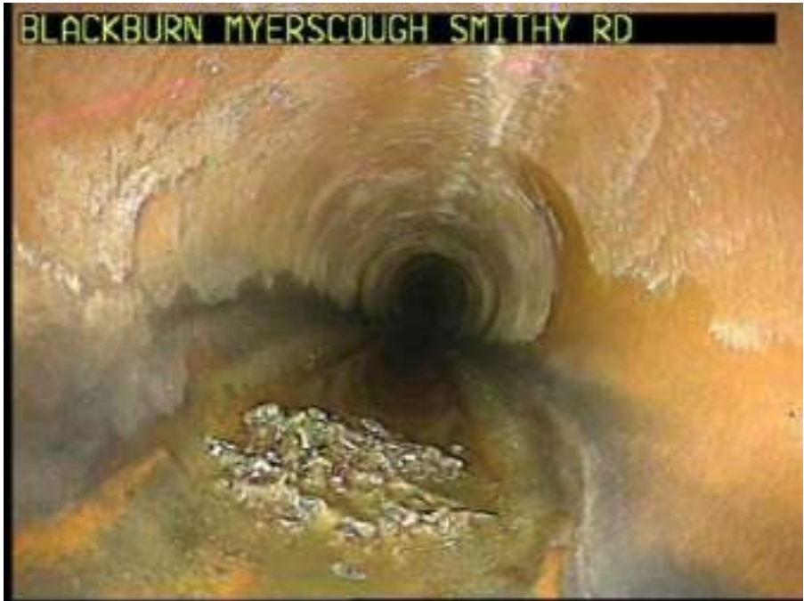
MH08AX_U_14082025_1232_067.jpg, 00:02:12, 23.79 m Settled deposits, coarse, 5% cross-sectional area loss
