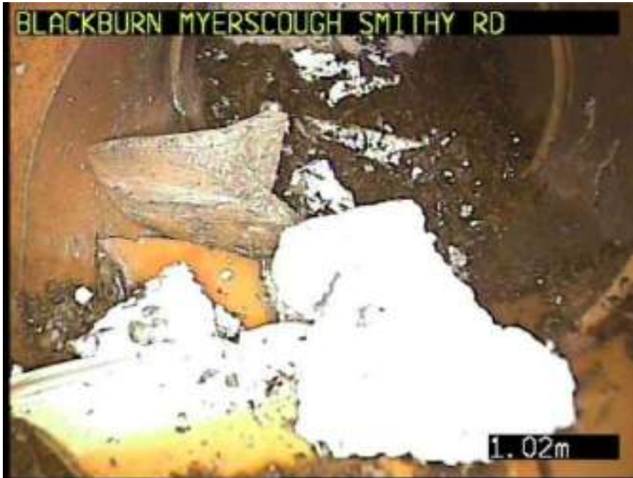
MH01AX_U_13082025_0954_008.jpg, 00:00:21, 1.02 m Settled deposits, other, 20% cross-sectional area loss, DEBRIS
