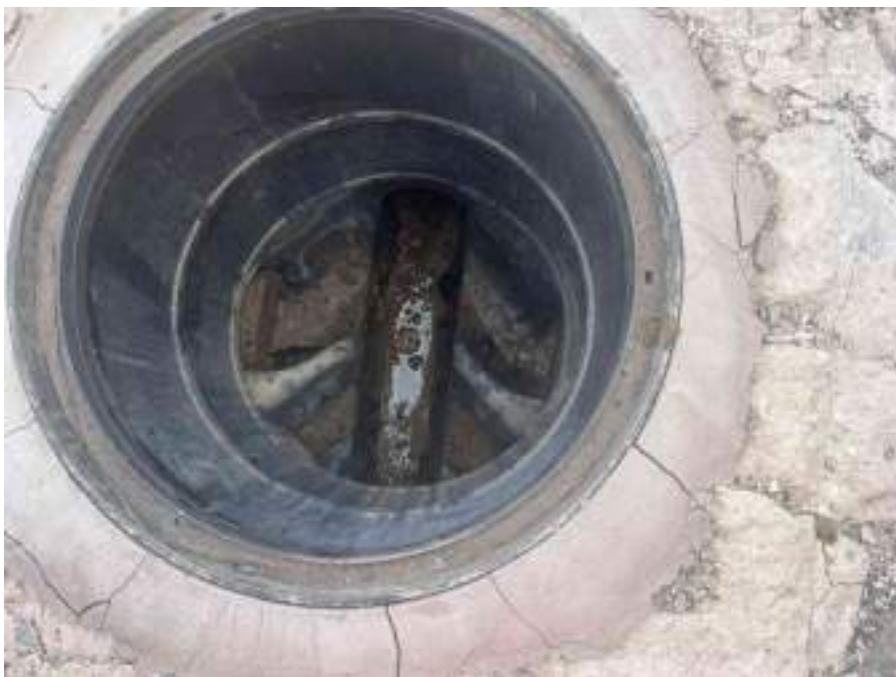
MH09X_D_14082025_1220_049.jpg, 00:00:00, 0.00 m Start node, inspection chamber, reference: MH09, IC LOCATED ADJACENT TO BAY DOORS
