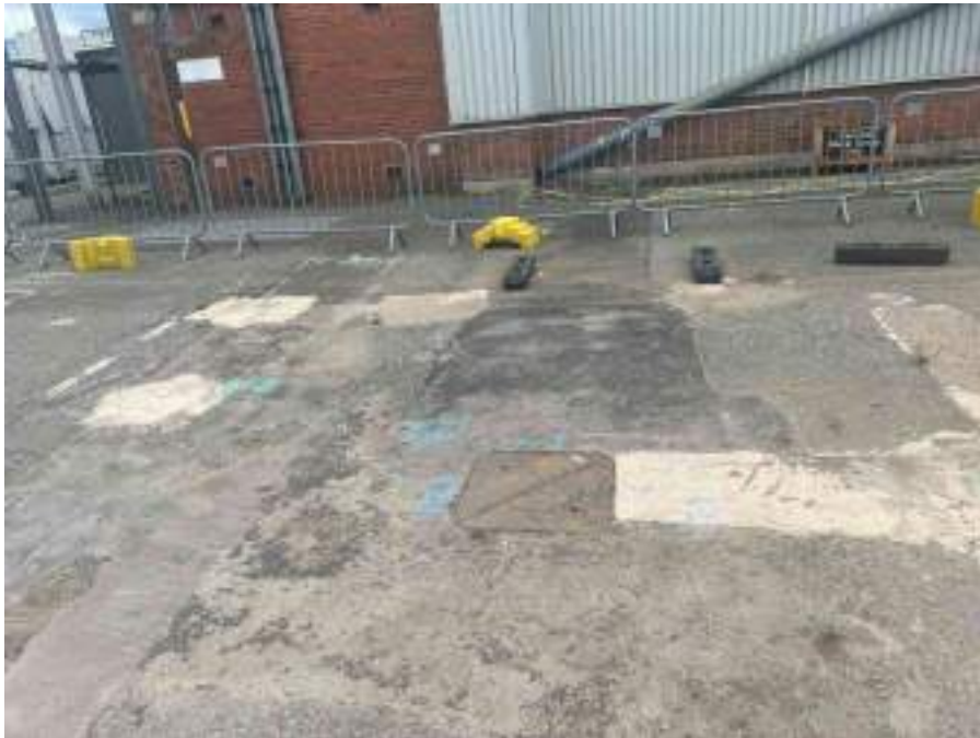
MH08X_D_14082025_1244_072.jpg, 00:00:00, 0.00 m Start node, manhole, reference: MH08, MANHOLE LOCATED ADJACENT TO LOADING BAY DOOR.
