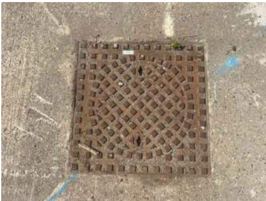
MH03X_U_13082025_1034_020.jpg, 00:01:47, 13.00 m Finish node, manhole, reference: MH03, MANHOLE LOCATED ADJACENT TO COOLING UNIT UTR
