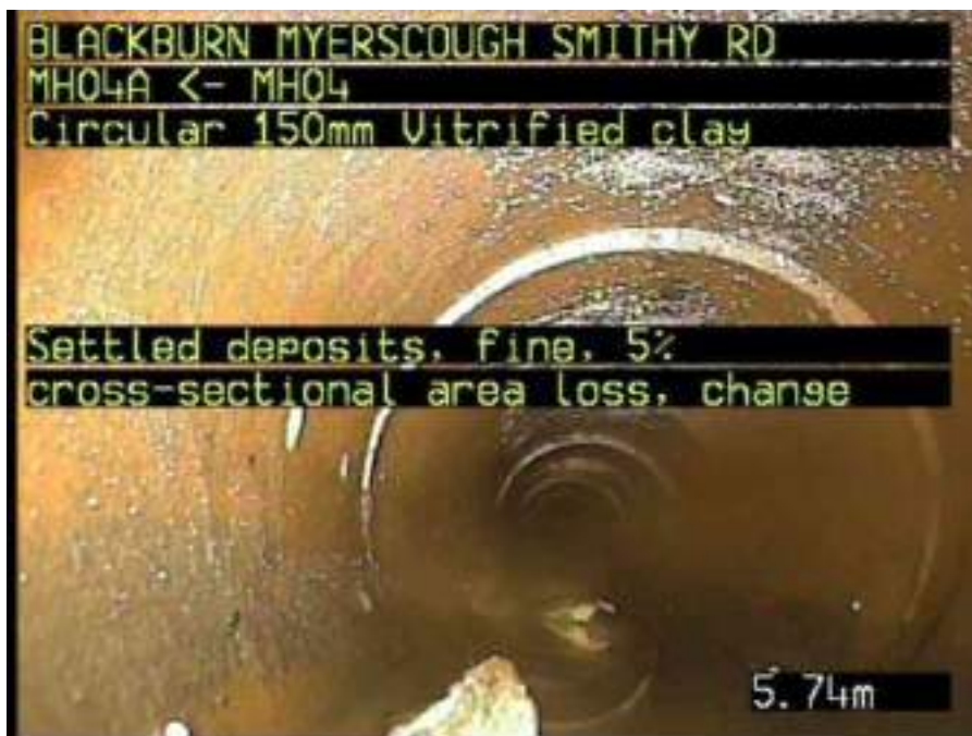
MH04AX_U_13082025_1217_042.jpg, 00:00:40, 5.74 m Settled deposits, fine, 5% cross-sectional area loss, change
