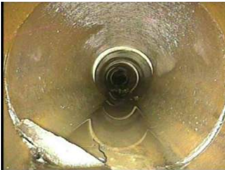
MH08X_D_14082025_1244_079.jpg, 00:03:47, 15.33 m Fracture, longitudinal at joint at 6 o'clock
