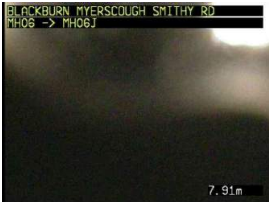
MH06X_D_13082025_1145_038.jpg, 00:00:57, 7.91 m Survey abandoned, CLEANSE REQ
