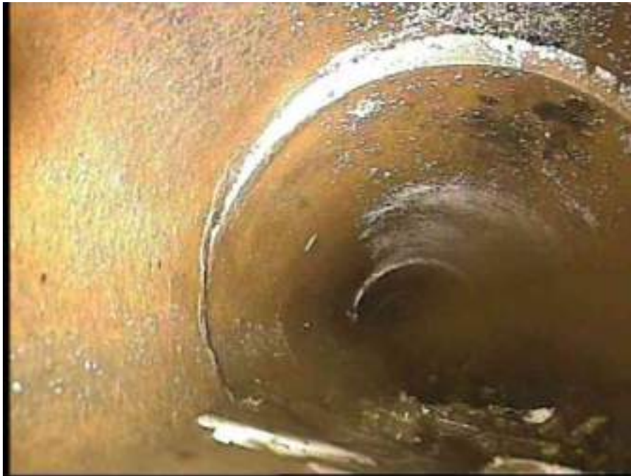
MH04AX_U_13082025_1217_043.jpg, 00:00:54, 7.22 m Settled deposits, coarse, 5% cross-sectional area loss
