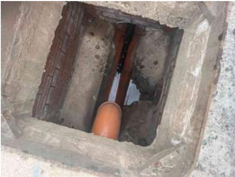
MH07X_U_14082025_1229_054.jpg, 00:00:00, 0.00 m Start node, manhole, reference: MH08, MANHOLE LOCATED ADJACENT TO LOADING BAY
