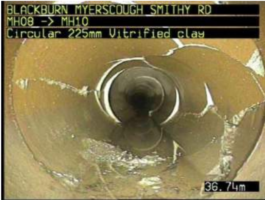
MH08X_D_14082025_1244_086.jpg, 00:06:57, 36.75 m Survey abandoned, UNABLE TO PROCEED WITH SURVEY DUE RISK OF EQUIPMENT OVER BROKEN PIPE
