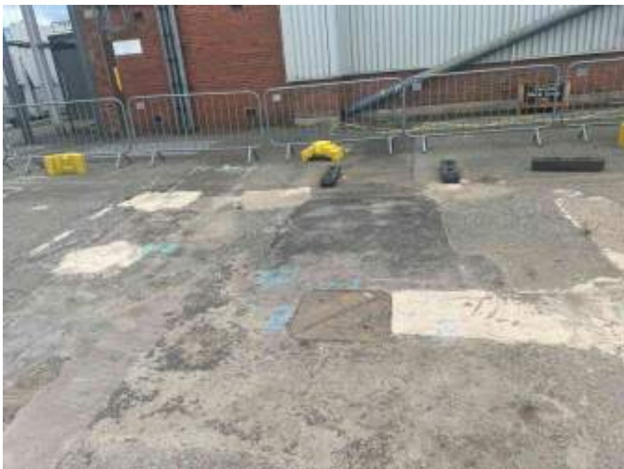
MH08AX_U_14082025_1232_064.jpg, 00:00:00, 0.00 m Start node, manhole, reference: MH08, MANHOLE LOCATED ADJACENT TO LOADING BAY
