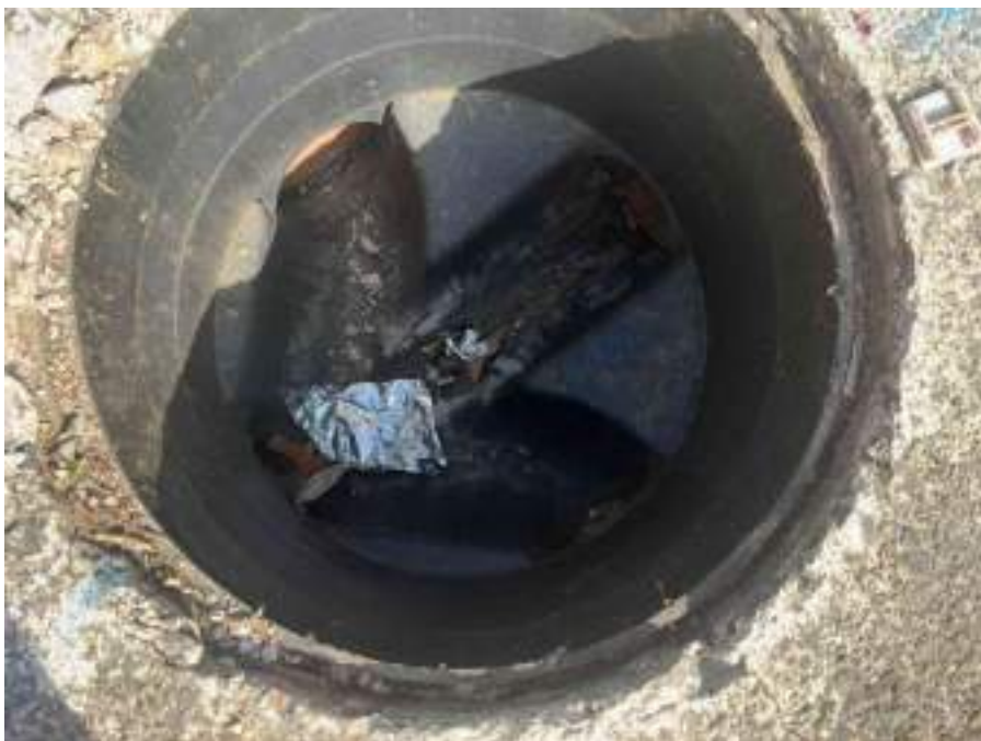
MH01AX_U_13082025_0954_007.jpg, 00:00:00, 0.00 m Start node, inspection chamber, reference: MH01, IC LOCATED ADJACENT TO STAIR CASE
