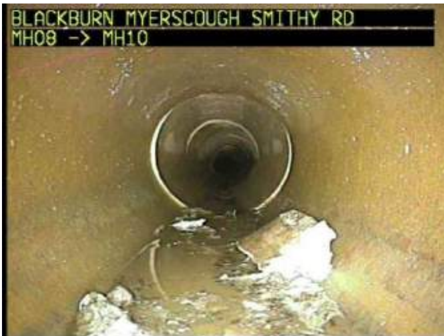
MH08X_D_14082025_1244_077.jpg, 00:01:24, 7.49 m Settled deposits, coarse, 10% cross-sectional area loss
