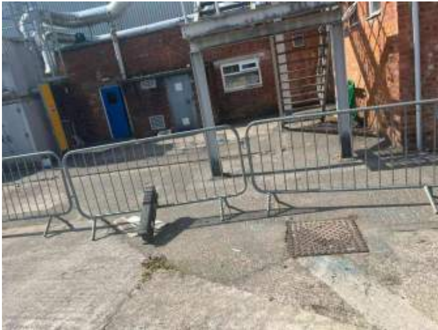
MH02X_D_13082025_1042_021.jpg, 00:00:00, 0.00 m Start node, manhole, reference: MH02, MANHOLE LOCATED ADJACENT TO STAIRCASE
