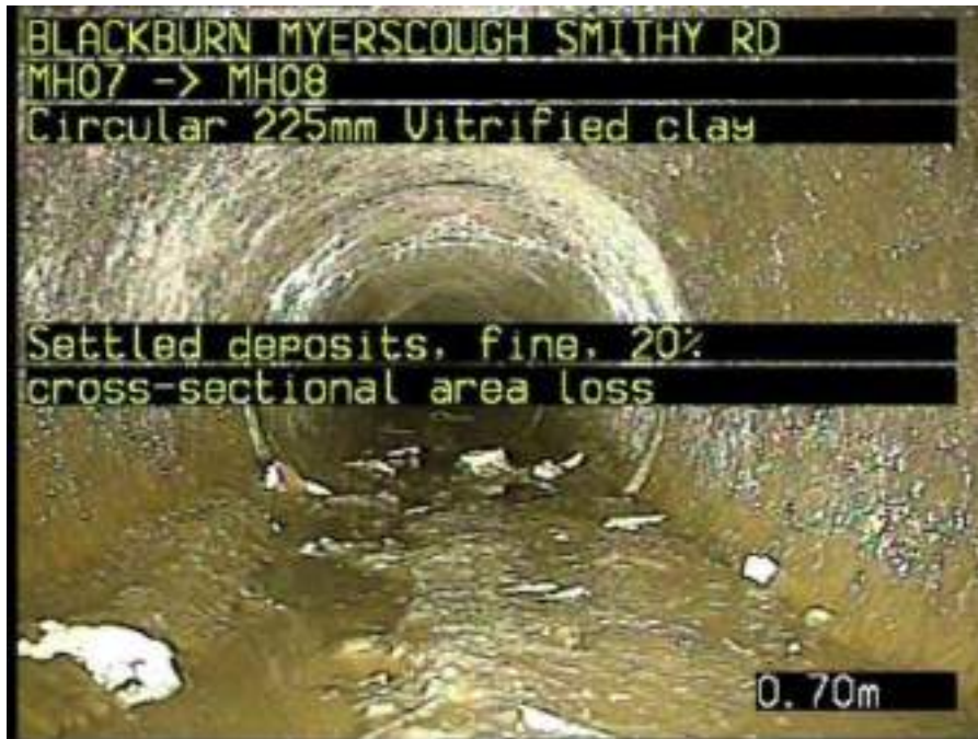
MH07X_D_14082025_1308_060.jpg, 00:00:05, 0.70 m Settled deposits, fine, 20% cross-sectional area loss, start
