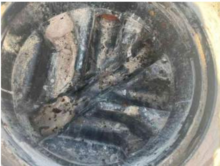
MH06X_D_13082025_1145_034.jpg, 00:00:00, 0.00 m Start node, inspection chamber, reference: MH06, IC LOCATED ADJACENT TO FILTER STORES
