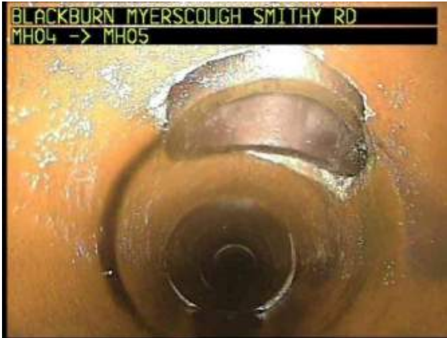
MH04X_D_13082025_1054_029.jpg, 00:00:54, 7.63 m Connection defective, connecting pipe is intruding at 12 o'clock, 100mm dia, intrusion: 5%
