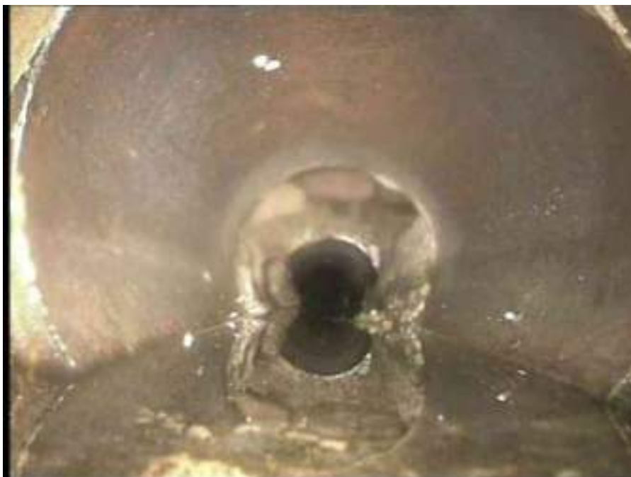
MH04X_D_13082025_1054_030.jpg, 00:01:27, 13.31 m Settled deposits, fine, 5% cross-sectional area loss
