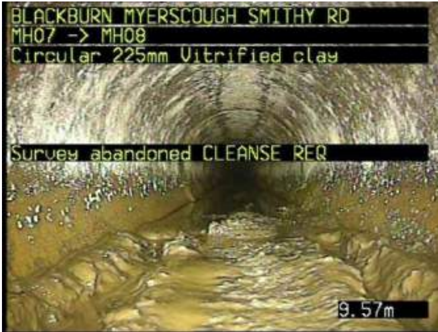
MH07X_D_14082025_1308_062.jpg, 00:01:37, 9.57 m Survey abandoned, CLEANSE REQ
