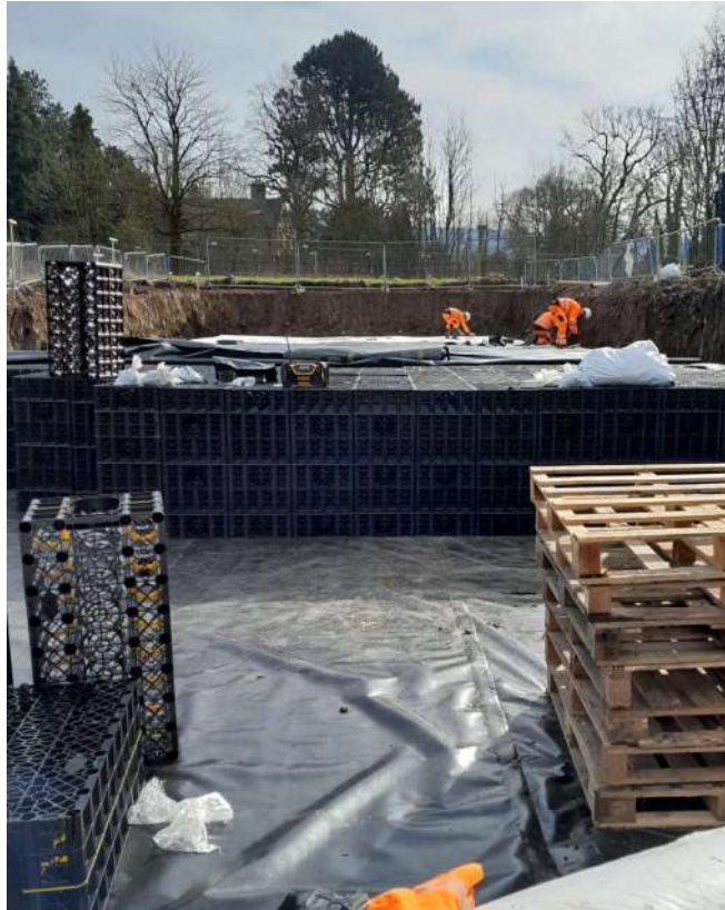
Photo 9 – proprietary “inspection” cells were placed in the bottom row as per specification
