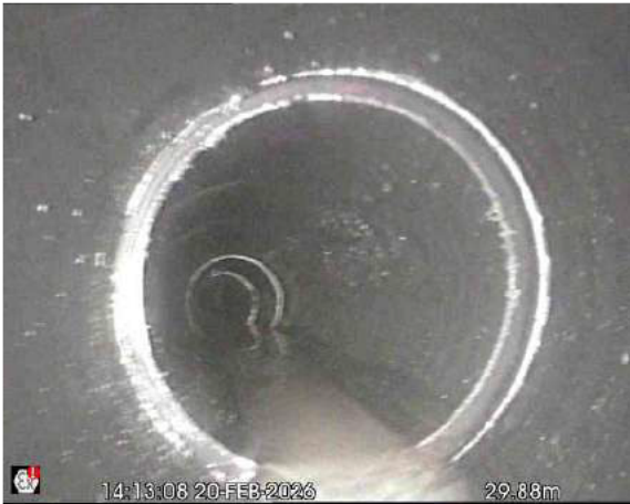
1, 00:02:17, 29.88 m Open joint, medium, Pipe deviates left on joint
