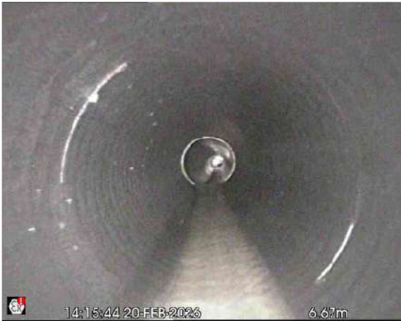
1, 00:00:38, 6.67 m General photograph taken at this point, possible crack
