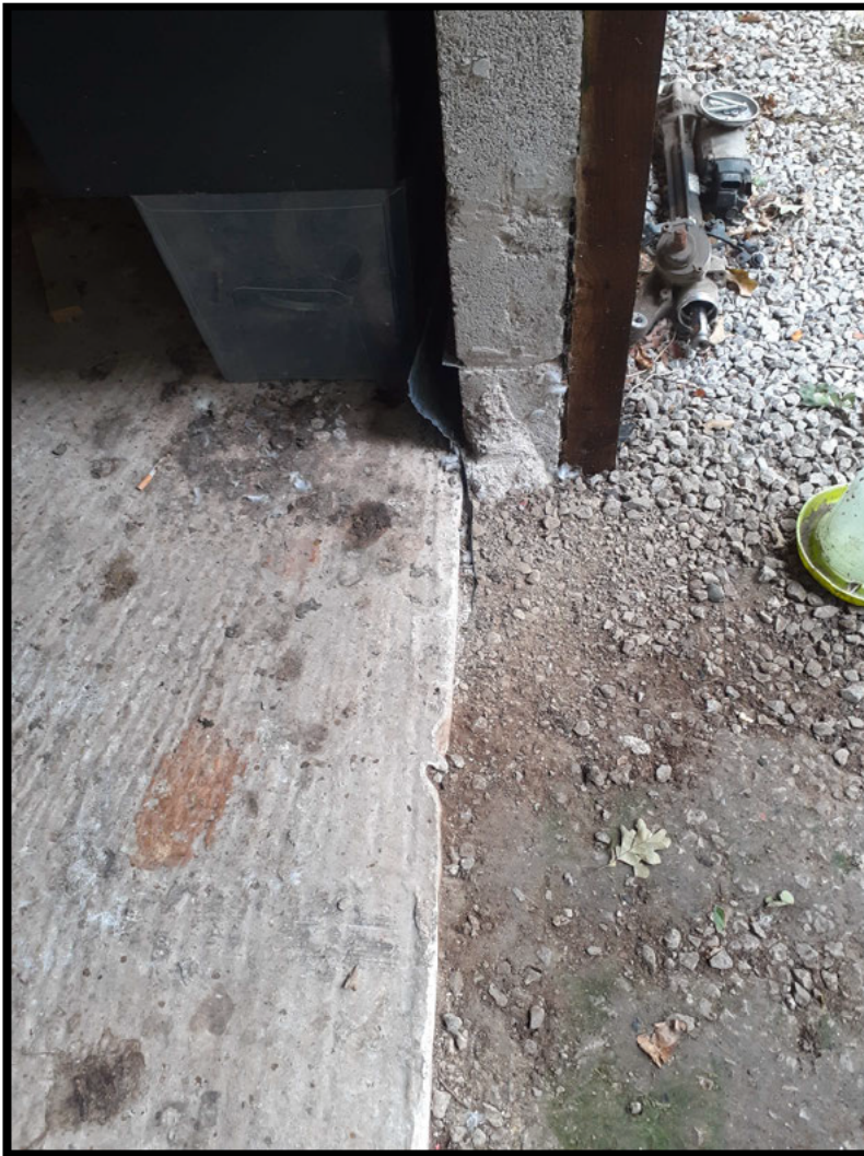
Ground floor and external wall showing damp proof course and damp proof membrane.
