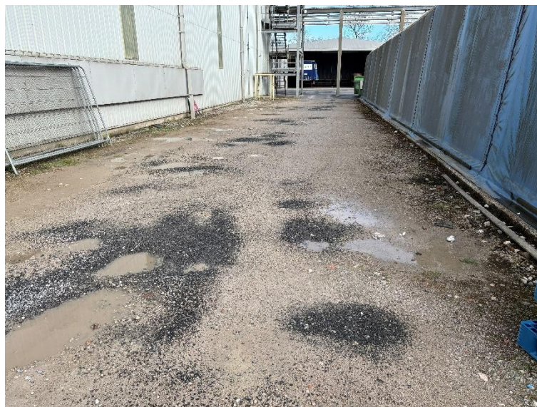
Photograph 3-4: An area of artificial, unvegetated, unsealed surface (u1c) in Site 1 - Main Control Room (B3)
