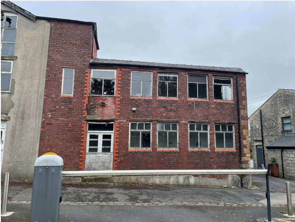
E7 – Brick Extension showing visible signs of deterioration.
