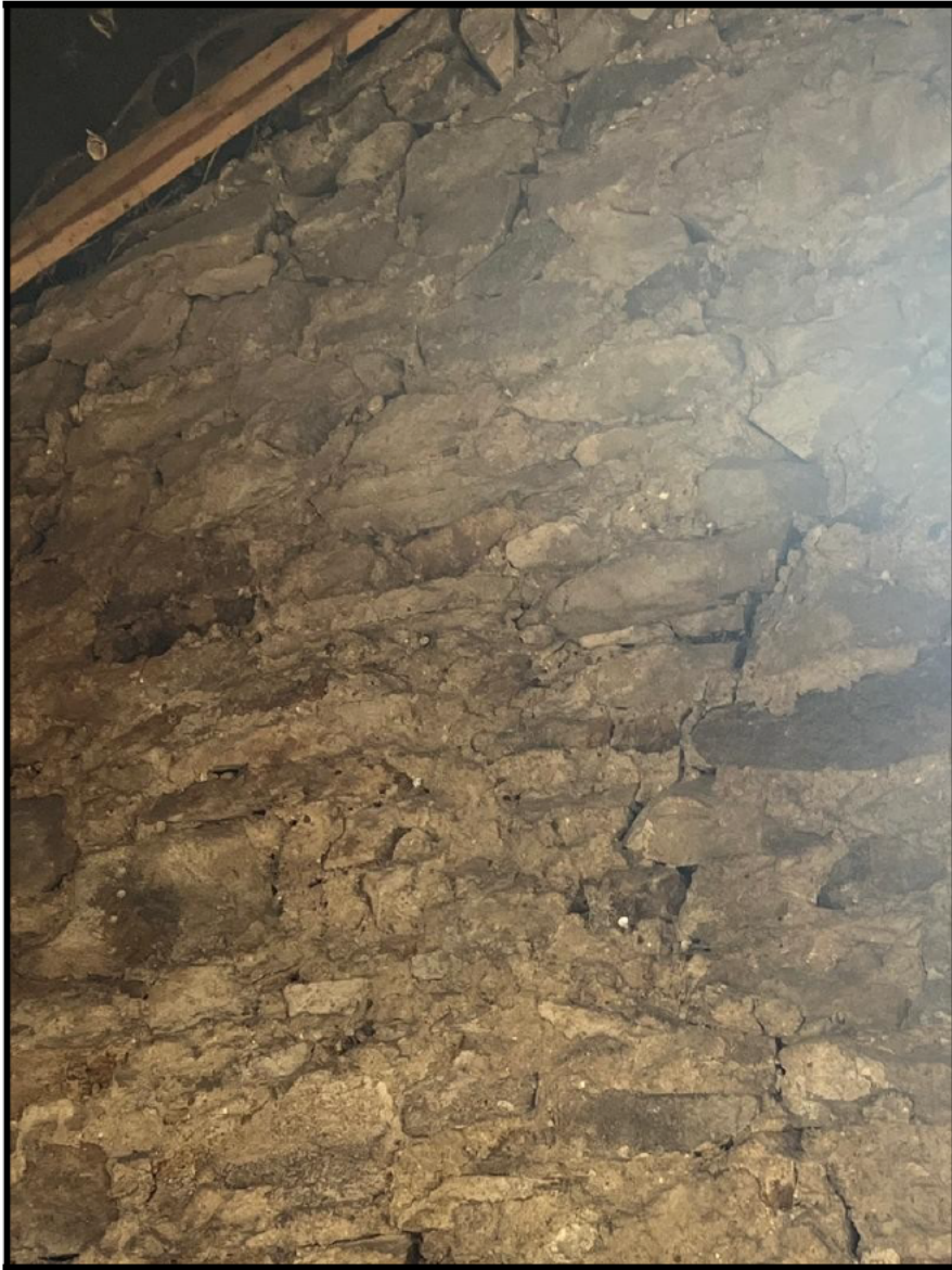
South gable wall showing movement cracks.
