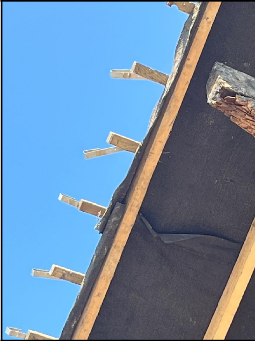
Exposed roof structure showing decayed purlin ends.
