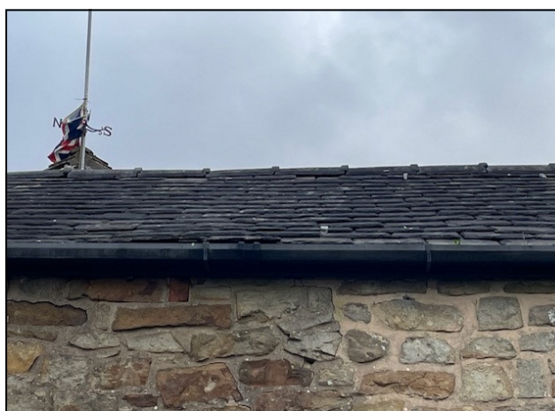
Plate 5 Gaps under roof coverings
