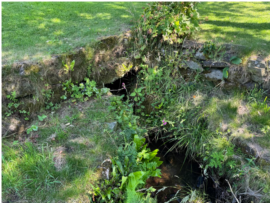
Fig 5 Tree roots and stones form obstructions within the culvert.
