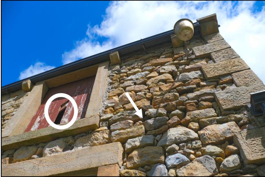
Image 8. Wall cavities in external walls. White arrow is the location of a second blue tit nest and the white circle is potential access for barn owl.
