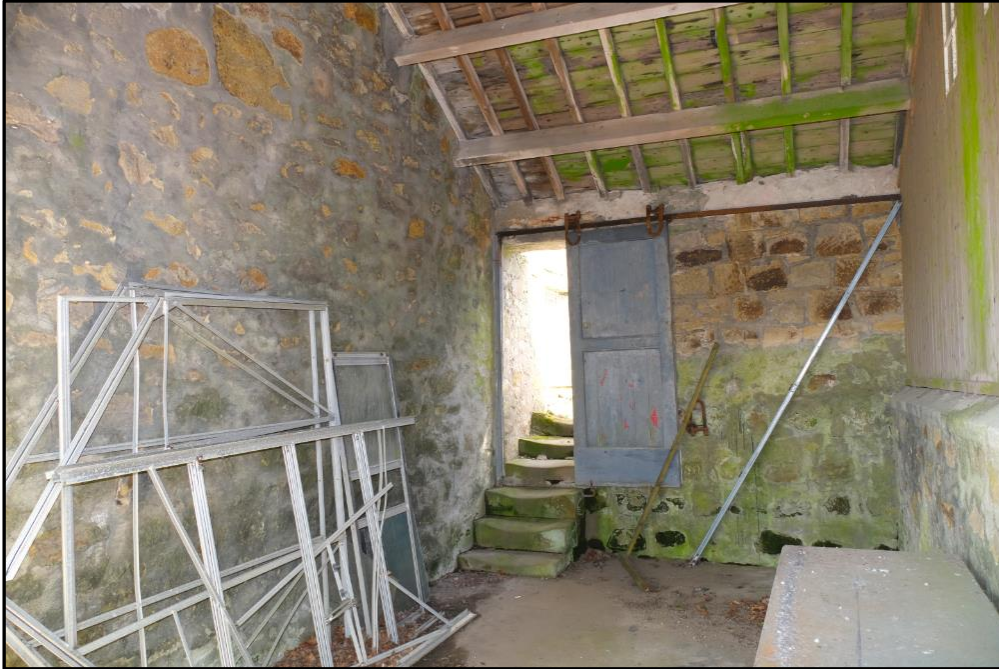
Image 5. Internal view of car port. There is clear evidence of past and current use by nesting swallows within timber under boarding and roof structures.
