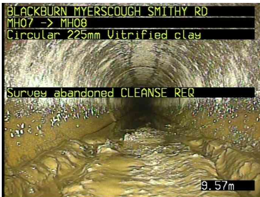
MH07X_D_14082025_1308_062.jpg, 00:01:37, 9.57 m Survey abandoned, CLEANSE REQ
