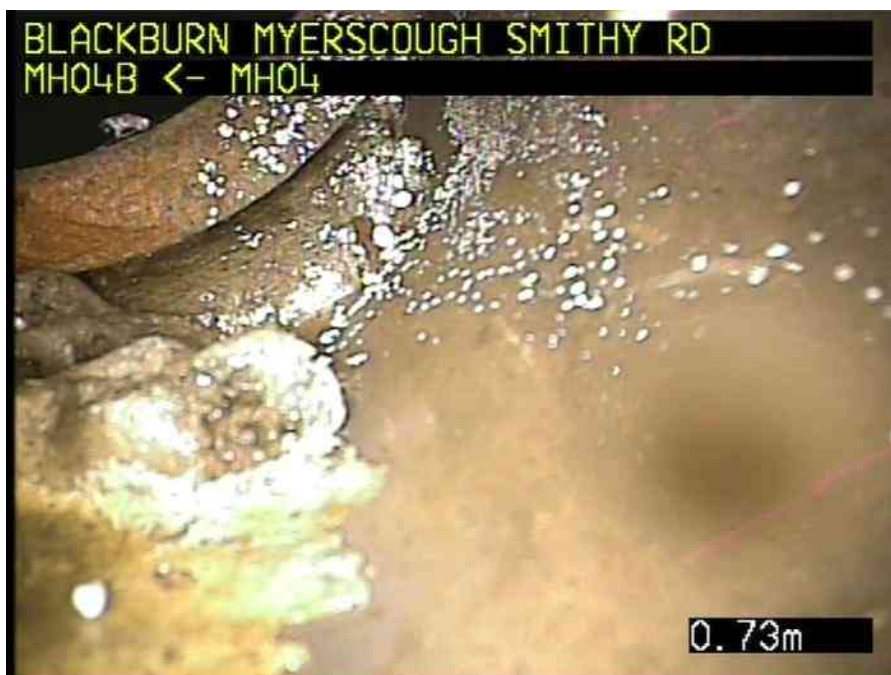
MH04BX_U_13082025_1225_047.jpg, 00:00:08, 0.60 m Joint displaced, large
