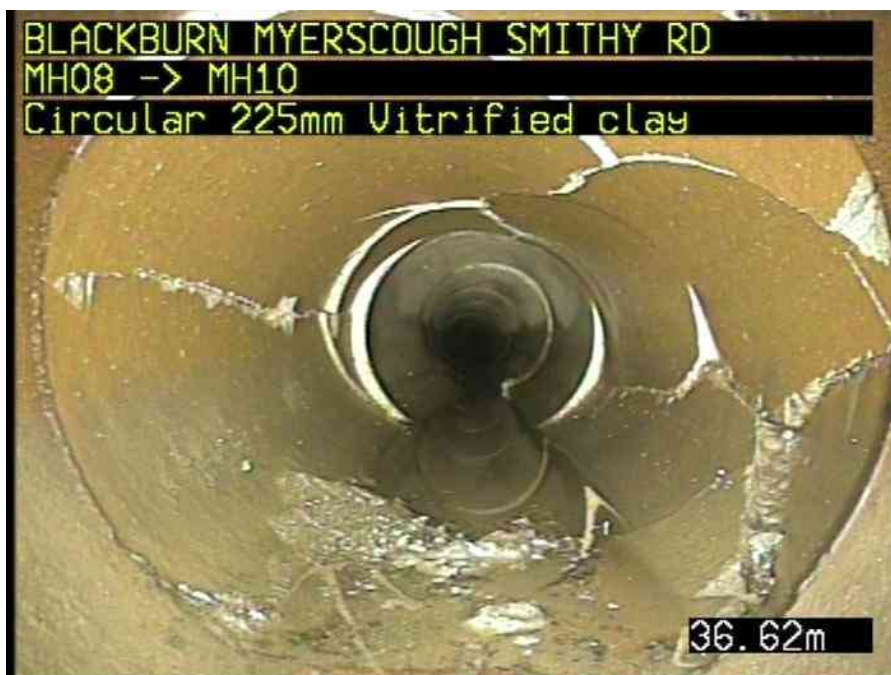
MH08X_D_14082025_1244_084.jpg, 00:06:45, 36.62 m Deformed sewer or drain, 10%
