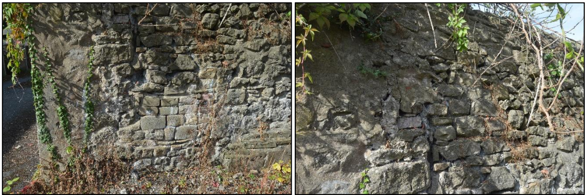
PL03: View of areas of perished mortar pointing.
