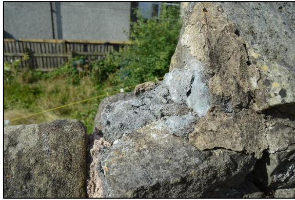
PL05: View of missing coping to the wall head increasing the risk of penetrating dampness.
