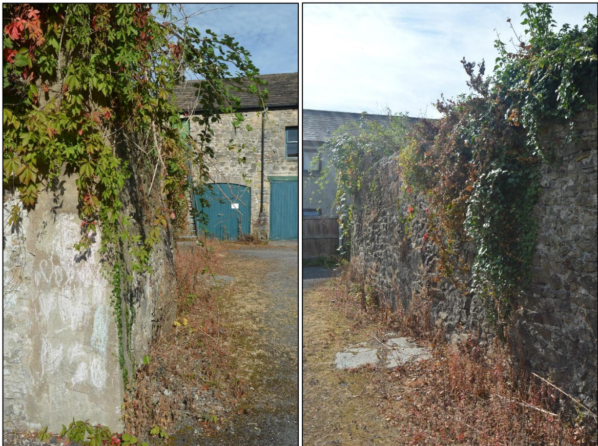
PL06: View of undulations noted along the length of the wall.
