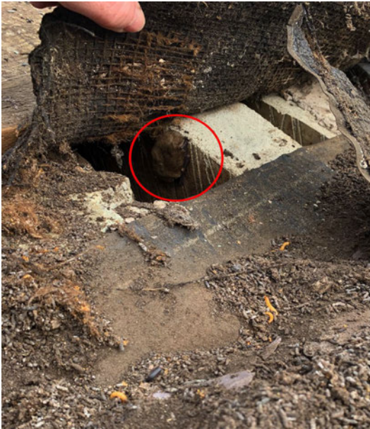
Pipistrelle bat below roofing felt.
